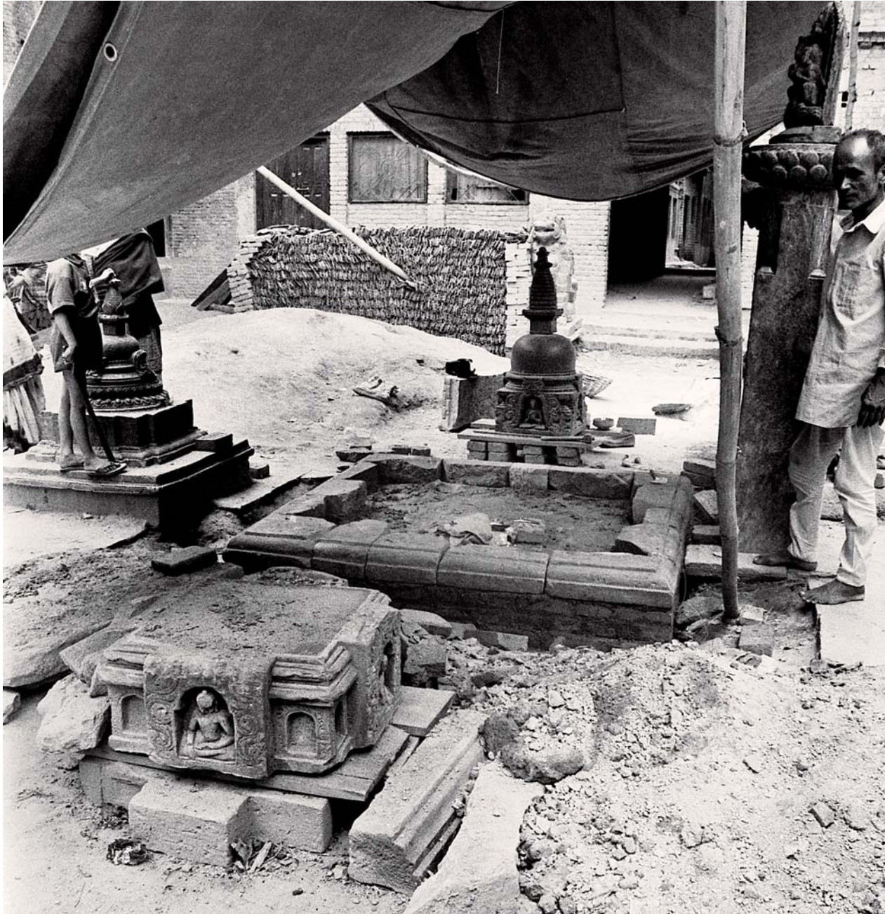
Vābhā, the Ratnanyāsa Pūjā Pannāratna Vajrācārya observes the offerings for the foundation of the caitya . Photograph by Nutandhar Śharmā, May 19, 1993.
