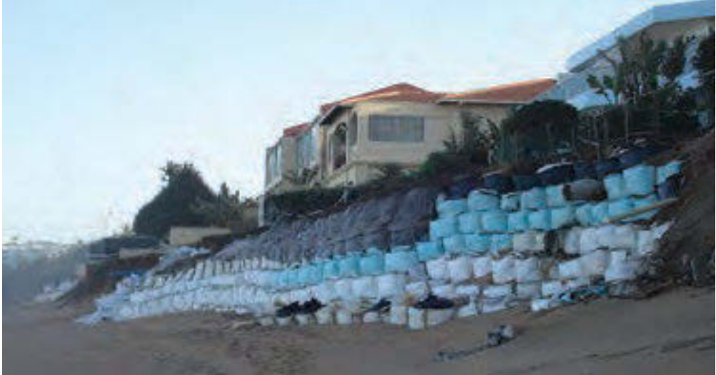
Figure 13.5. Damage to the beach, property and infrastructure following a spring-high-tide storm surge, Ballito, KwaZulu-Natal, 2007.
