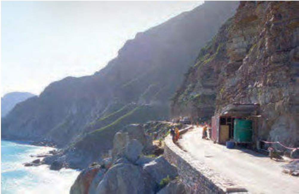
Figure 13.3. Refurbishment of Chapman's Peak Drive in 2003. The original road follows the unconformable contact between granite (below the road) and inherently unstable Graafwater Formation mudstones and sandstones (above the road).
