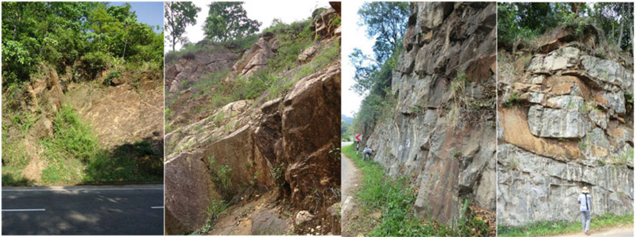
Fig. 20 Example of rock formed failures along the road side slope. Wedge failure, translational slides and falling rocks are very much significant along the road sides. High hazard potential zone can be observed due to foliated and jointed rock formations (Fig. 13 in Dias et al. 2022)
