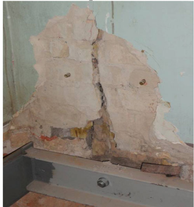
Fig. 3 Vertical crack with a width of up to 2.0 cm
