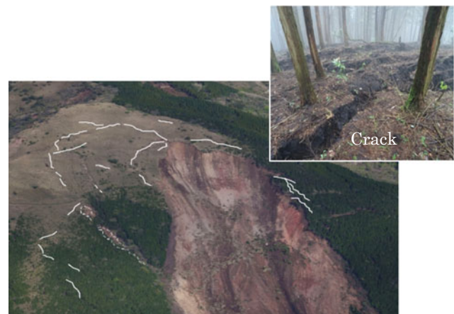
Fig. 11 The head part of the slope failure and the distribution of cracks around the failure (upper) and the cracks around the failure (white line: lower) (Photo: Kyushu Regional Development Bureau, MLIT 2016)
