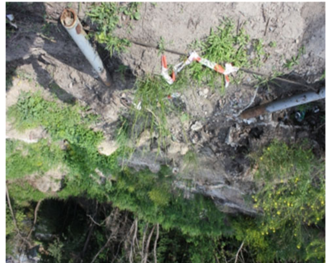
Fig. 2 An example of the active development of landslide processes with active developments and erosion processes on the slope of the Church
