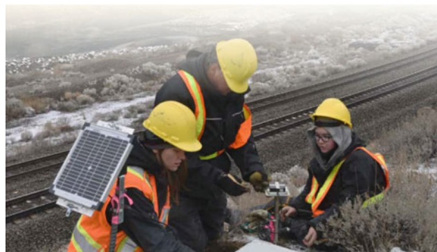
Fig. C.5 The GSC conducts geohazard studies to reduce risks to people and infrastructure, here installing equipment to monitor landslide activity above a critical railway corridor in central BC
