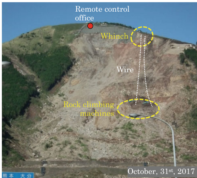
Fig. 14 Removal of unstable sediment by unmanned construction (Modified from source: Kyushu Regional Development Bureau, MLIT 2020)
