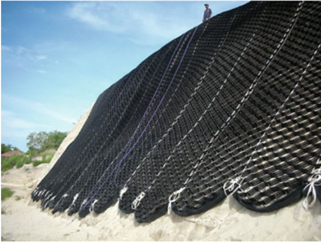
Fig. B.1 Geosynthetics used to stabilize a slope using soil in-fill and seeding for plants
