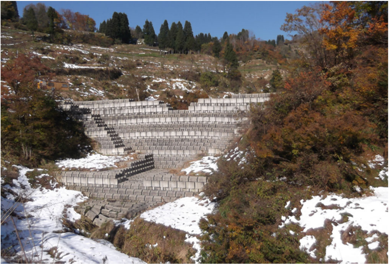
Fig. 12 Azumagawa Check Dam at N 37.3300°, E 138.9021°. The center of the dam crest was 0.4–0.5 m higher than the abutments as of November 17, 2013
