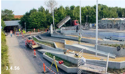
3.4.51–3.4.52 Rounded shapes of the relief at the competition stage. Redrawn from the competition plan 3.4.53–3.4.54 Rectilinear forms of the relief as realized resonating with the surface pattern. Redrawn scheme from aerial photograph of the completed project 3.4.55–3.4.56 Retaining walls delimiting containers
