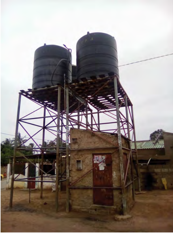
Fig. 5: Water storage tanks of a private water supplier in the district of KaMubukwana, Maputo (S. Thomschke [2019]).
