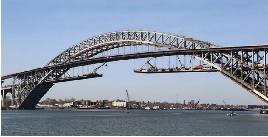
Fig. 7.8. Construction underway at the Bayonne Bridge to raise the bridge's clearance by sixty-four feet. The original deck has yet to be fully removed in this photo. (Photograph reprinted by permission of Port Authority of New York and New Jersey.)
