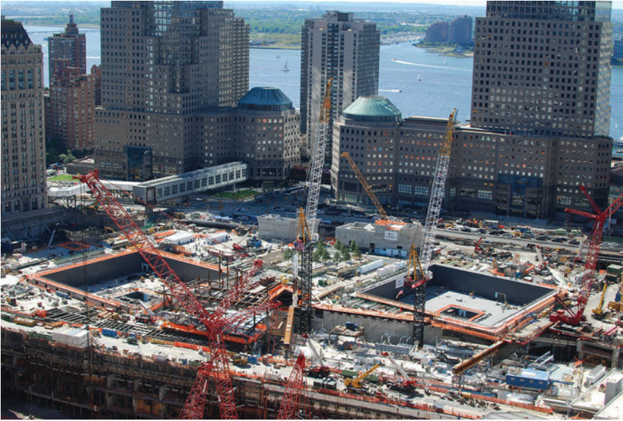
Fig. 8.9. Construction of the National September 11 Memorial & Museum in 2010. (Photograph by Derek Rose, September 11, 2010. Courtesy Wikimedia Commons, CC BY 2.0.)
