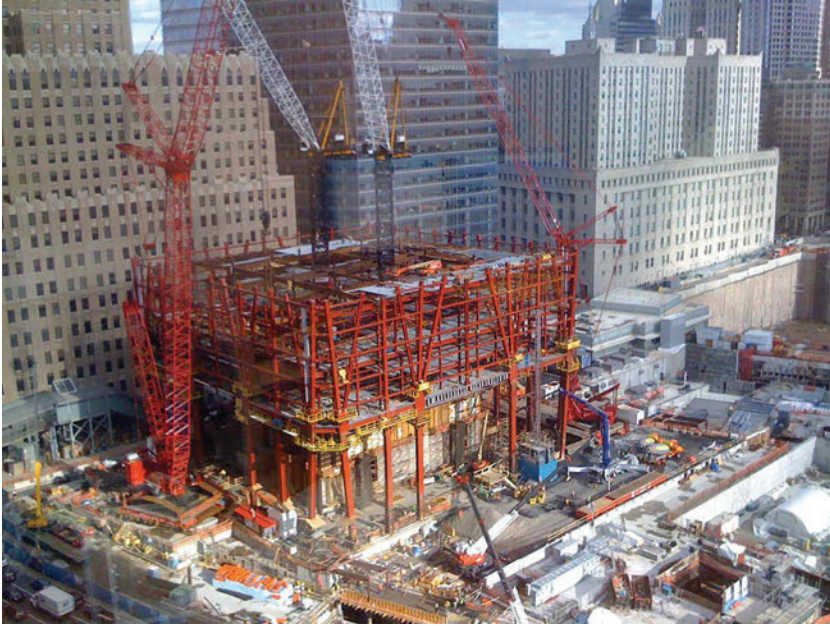
Fig. 8.8. Construction of One World Trade Center (Freedom Tower) in 2009. (Photograph by Westmc9th, December 2009. Courtesy Wikimedia Commons, CC BY-SA 4.0.)
