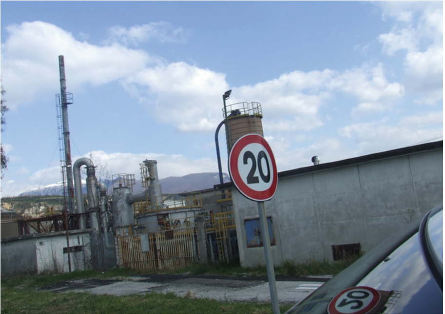
Fig. 4. Plants of the purification sector.
