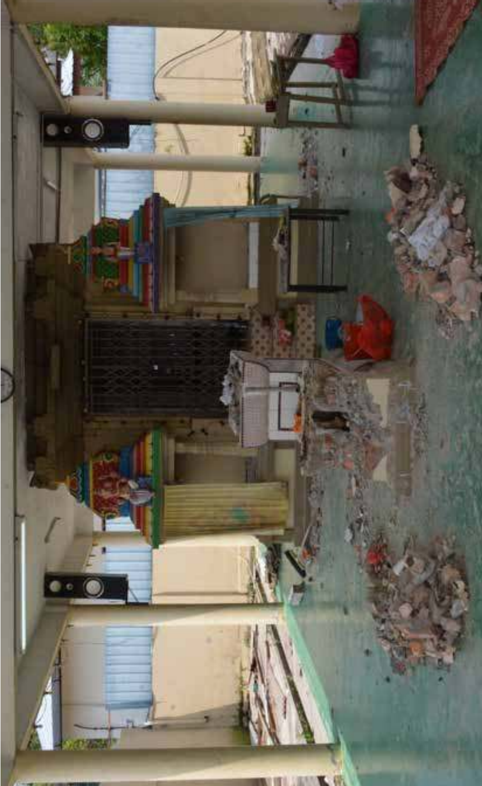
Figure 6.2. Demolition in progress, the Sri Maha Mariamman Temple, Mengkibol, 2017. © Ravinran Kumaran, used with permission
