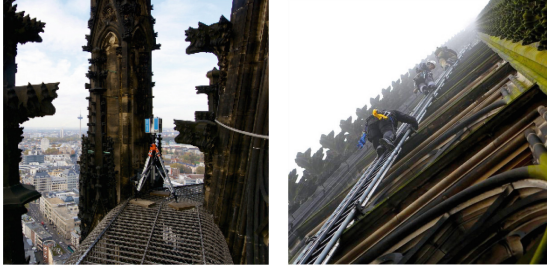
Fig. 14. Exposed logistics on the exterior of a tall gothic spire (Cologne Cathedral) 2 .
