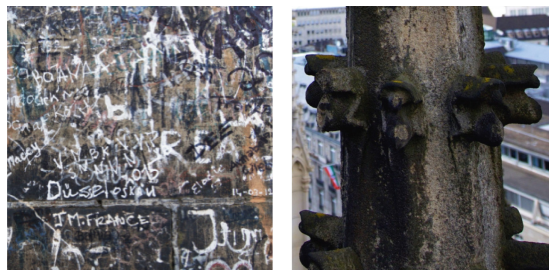
Fig. 13. Factors of survey data alteration: vandalism and surface flora at Cologne Cathedral 2 .
