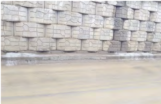
Figure 3. Escape of the fly ash fines from the fascia of the RE wall.
