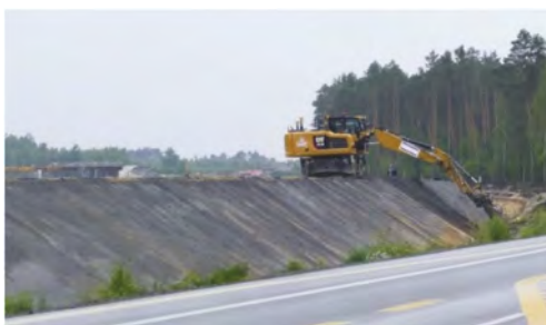
Figure 2. Forming a slope from ashes on the section Janów Lubelski – Łązek of the S19 expressway in Poland (May 2020) (GDDKiA).
