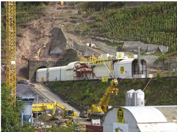
Figure 3-5. Mobile TES installed on fixed housing.
