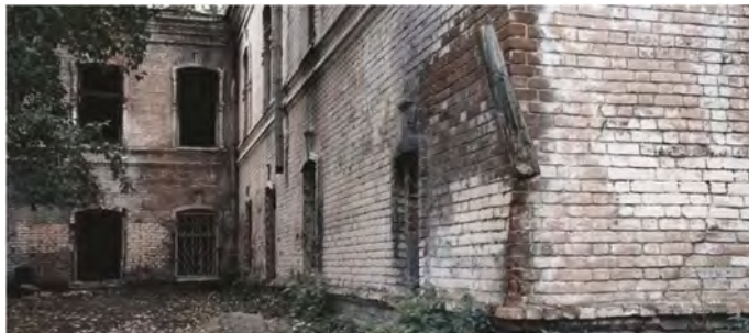
Figure 1. “Tekutievo hospital” before restoration (2011).
