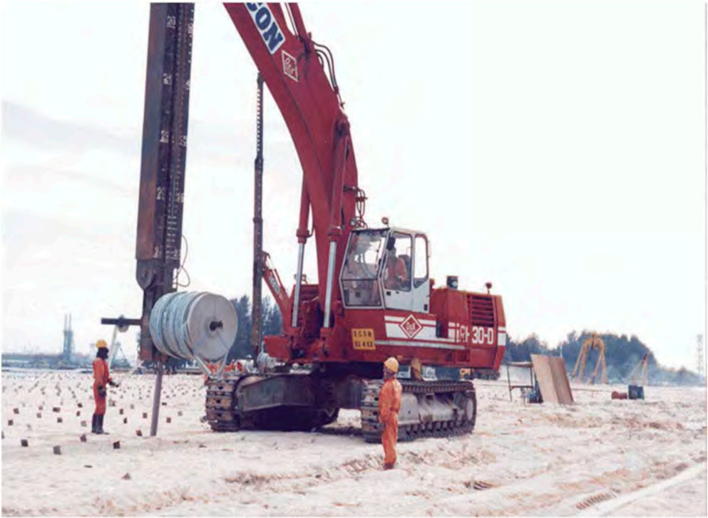
(a) Flexible band drains being installed in reclaimed land (photograph courtesy of Prof. Jian CHU)
