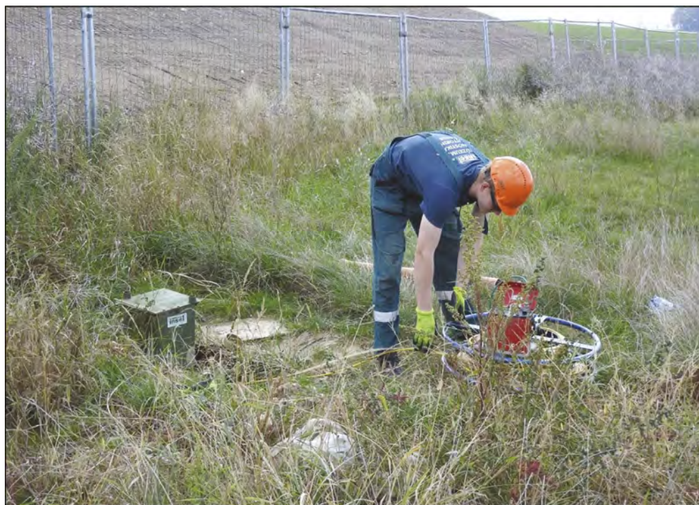
Figure 3. Hydrostatic levelling – all measured data were continuously available on portal https://inset.sahure.cz/Sahure .
