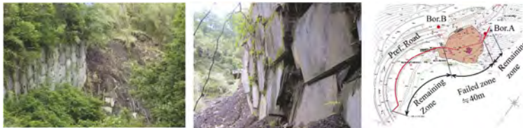
Figure 2. Condition of remaining and collapsed reinforced soil wall and plane alignment of wall.
