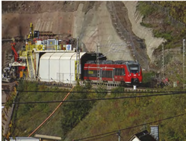
Figure 1. The Petersberg rail tunnel will be refurbished by late 2019 by the tunnel-in tunnel method while rail services continue.
