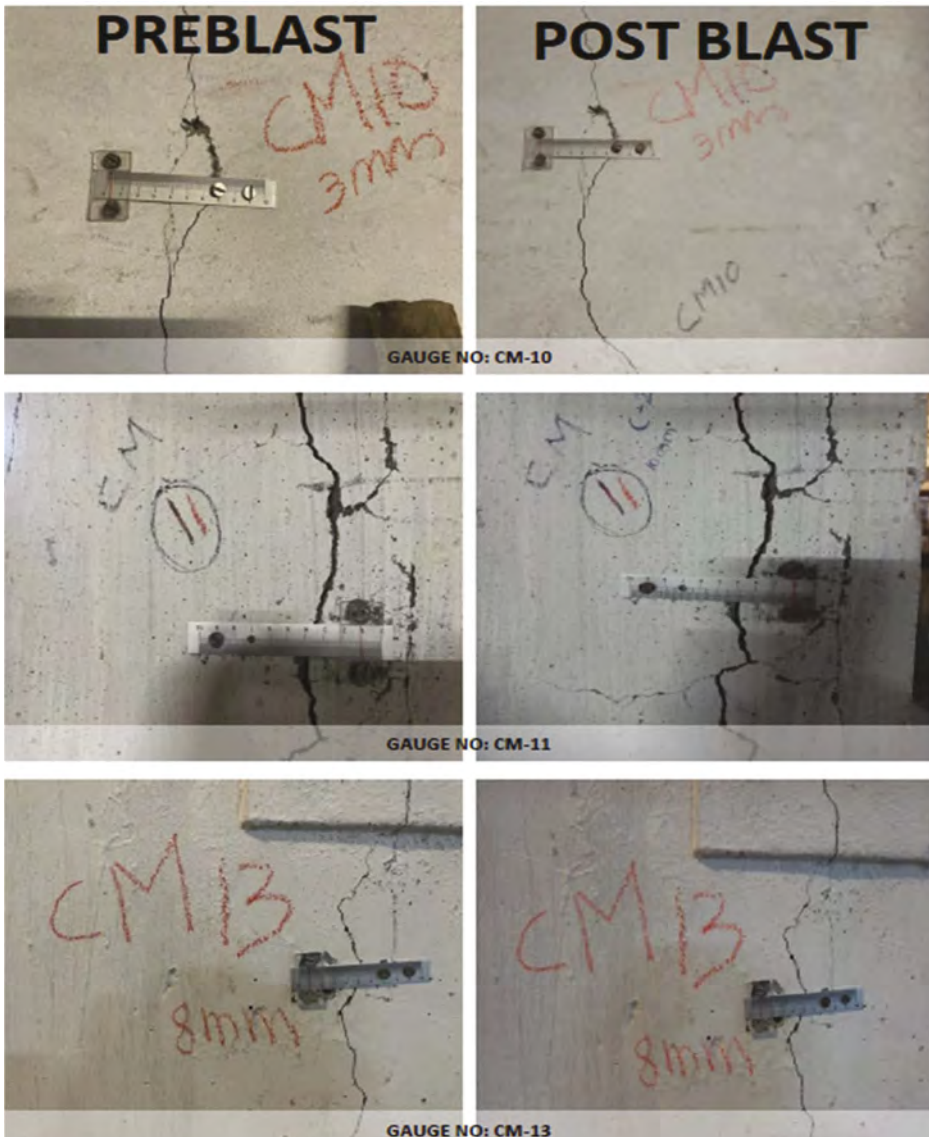
Figure 10. Crack meter reading pre and post blast.
