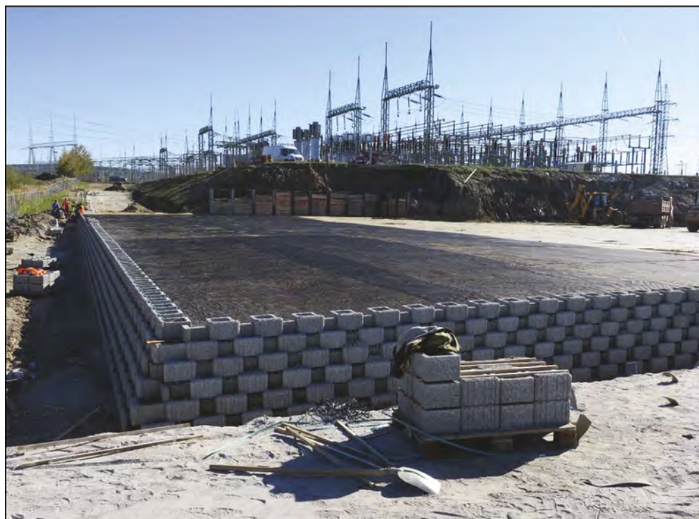
Figure 1. Construction of the embankment in process (high voltage transformer in the background).
