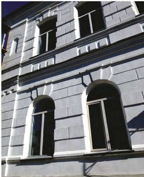
Figure 4. The building of the Kazakh Humanitarian Law Innovative University, after restoration (fragment).
