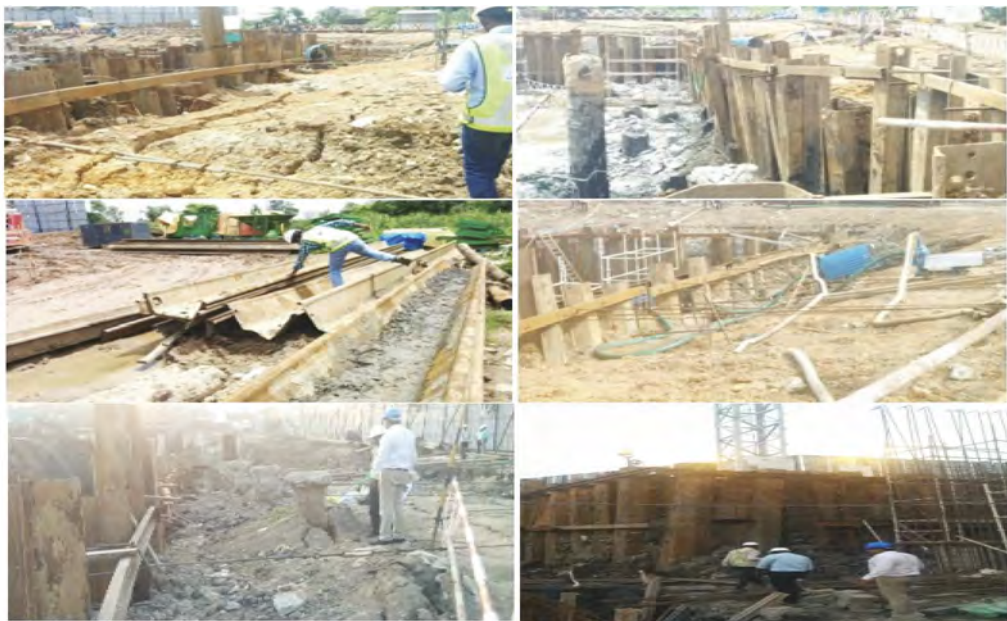
Figure 8. Huge stress on sheet piling system due to block movement of the soft clay.
