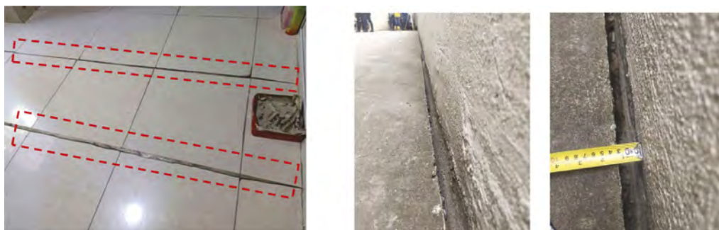
Figure 6. Reported damages: (a) damaged floor tiles & (b) lateral displacement of perimeter wall.
