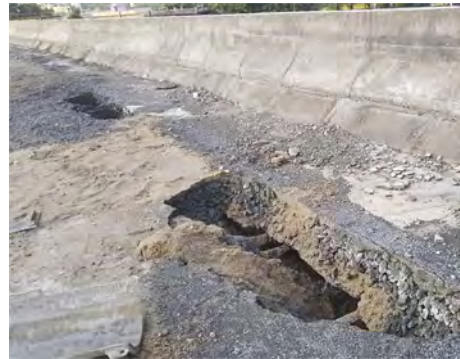
Figure 4. Large potholes at various locations on the flexible pavement.
