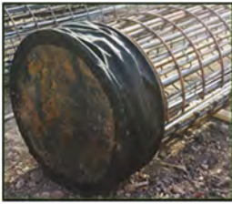
Figure 3a. Photograph of a smart cell attached to the bottom of a steel reinforcement cage.
