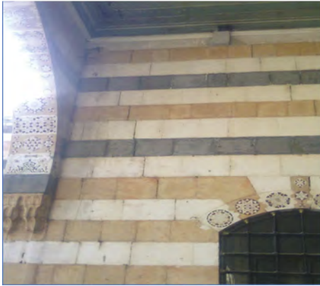
Figure 3. Cracks in Al-Azem Palace.
