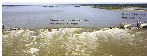
Figure 1. Breached portion of the regulator at Upper Anicut (Image courtesy: The Hindu, 2018).
