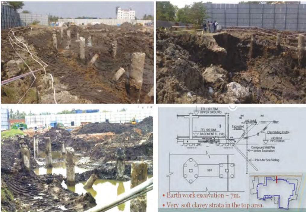
Figure 6. Failure of stage excavation.
