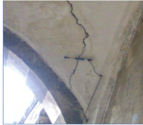
Figure 4. Cracks in the cupolas.
