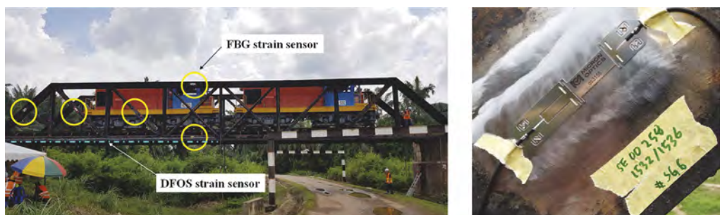
Figure 3. Application of DFOS and FBG sensors for 100-year-old bridge's static and dynamic assessment.
