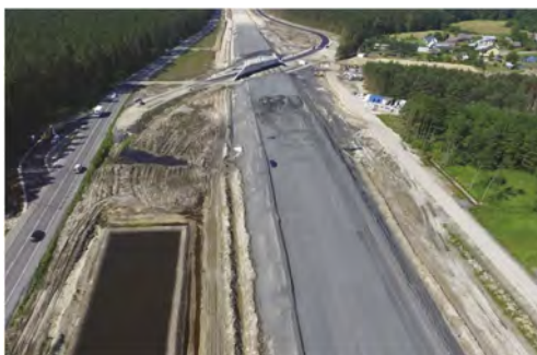
Figure 3. View from above on the S19 expressway embankment, made of ashes from the combustion waste landfill “Jelnia” (May 2020) (GDDKiA).
