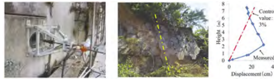
Figure 3. In situ pull-out test and displacement measurement of wall facings by laser rangefinder.
