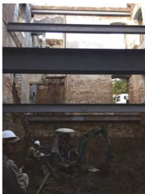
Figure 6. Work process: installation of tie girder for the basement floor; excavation of the soil to the depth of the underground floor.
