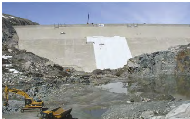
Figure 8. Rehabilitation of Midtbotnvatn rockfill dam in Norway: placing of PVC composite geomembrane layer over the damaged cement concrete facing.
