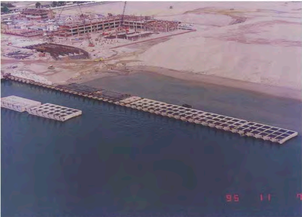
(b) Surcharge works on reclaimed land for the construction of Pasir Panjang Container Port Phase 1
