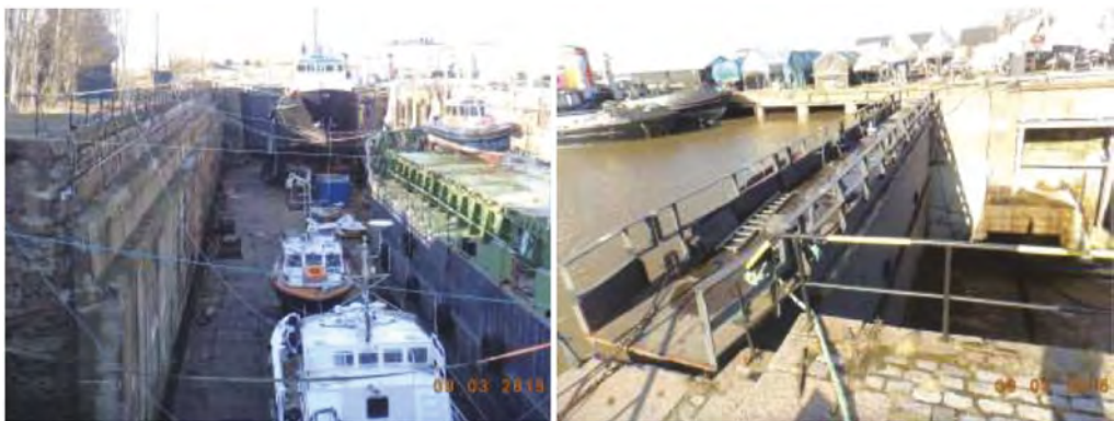
Figure 1. Dry dock of Suomenlinna and strengthened corner of the floating door.
