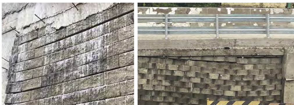
Figure 1. Fascia settlement of RE wall-1 by 25 mm. Figure 2. Fascia settlement of RE wall-2 by 65 mm.
