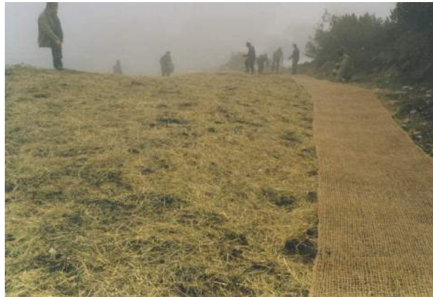
Figure 8: Geotextiles are used predominantly where site conditions are extreme, particularly at sites with danger of erosion (Lawinenstein, Austria, 1800 m a.s.l.).
