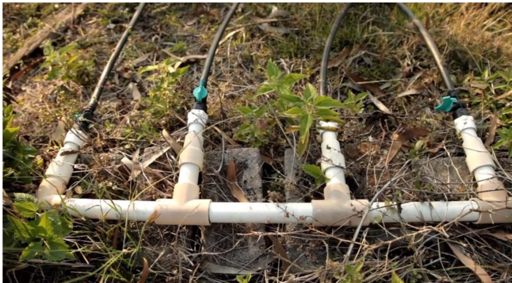
Figure 16. Water distribution pipes for drip irrigation.
