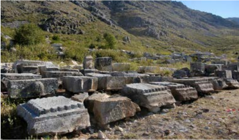
Fig. 10. Blocks recorded and removed from the trench are organised on a stone platform.
