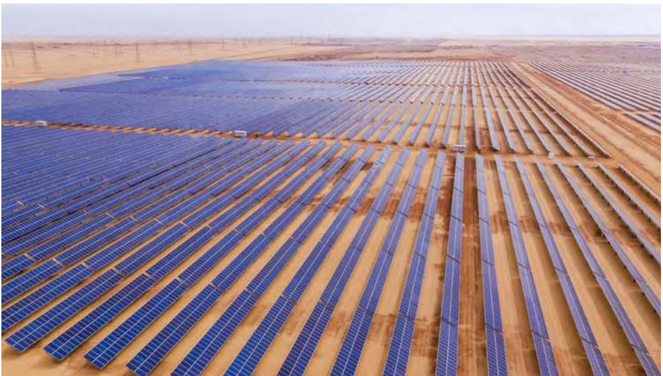
Benban solar park, Egypt. The EBRD took a major step forward to support the rollout of renewable energy in Egypt in 2017 with the approval of a US$ 500 million framework to support the development of Benban, the largest solar park on the African continent. © EBRD
