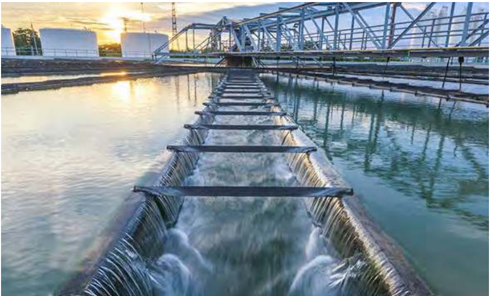
In Skopje, North Macedonia, wastewater treatment has been identified as one of the most urgent tasks under the Green Cities Action Plan developed by the city authorities and the EBRD. © EBRD
