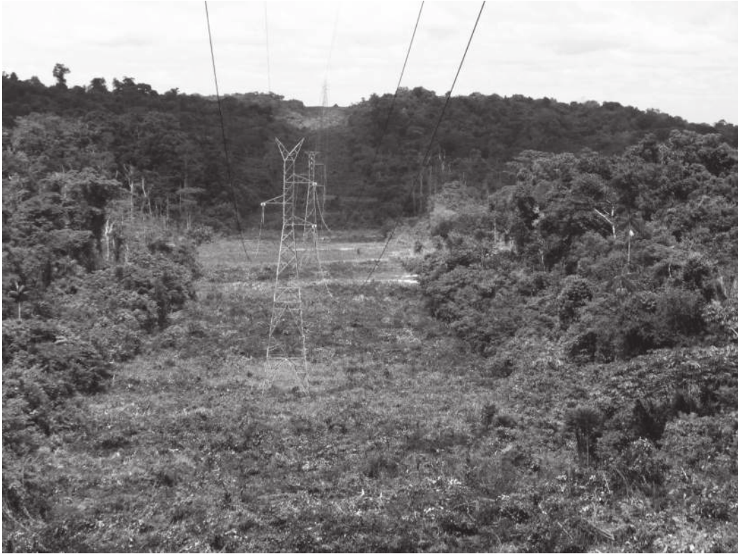
Figure 4.6 The functioning power line, outside the north-west boundary of Canaima National Park (Photo by Iokiñe Rodríguez)
