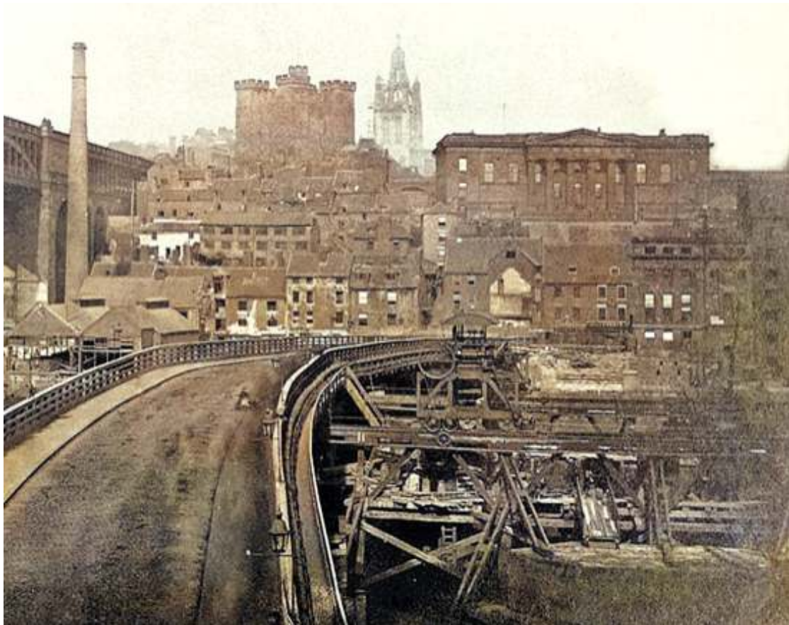
Figure 4. The Georgian bridge during demolition to make way for the Swing-Bridge, 1871-2. As viewed from Gateshead looking north towards the Castle and St. Nicholas's Cathedral. Peeping through the thicket of scaffolding and machinery is perhaps the very ladder Bruce descended to reach the bed of the river. To the left is the gas-lit temporary bridge built in 1866. Removing the debris of the Georgian Bridge has left the soot-stained building facades behind coated with wind-blown sandstone dust (© Newcastle City Library, Local Studies Collections Accn No. 046776).
