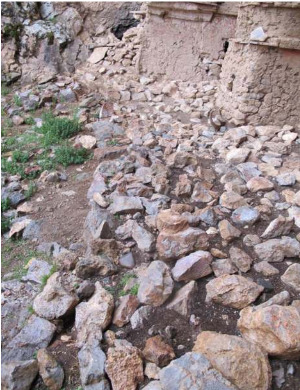
Figure 305. The trio of built chortens were placed on a wide masonry platform. Despite being highly degraded, this structure can clearly be seen elevated above the floor of the overhang.
