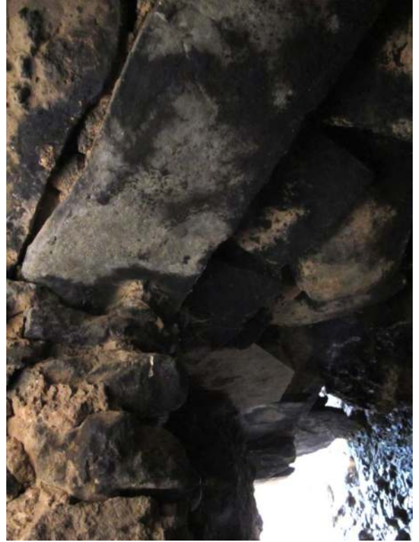
Figure 312. A view of the corbelled ceiling over the chamber created by the twin chortens erected at Chu ro.
