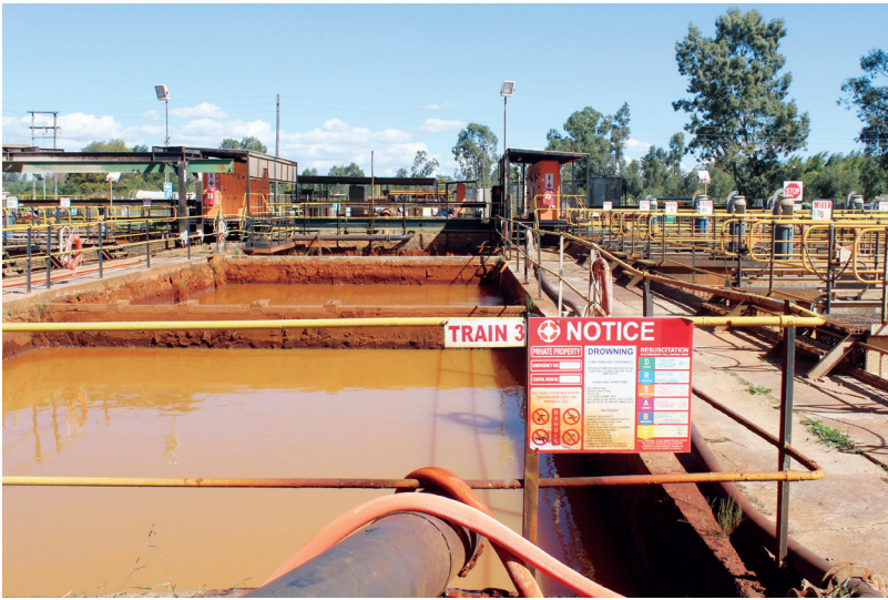
2.12 Western Basin AMD Treatment Facility, 2022. Luka Edwards Hecht.
