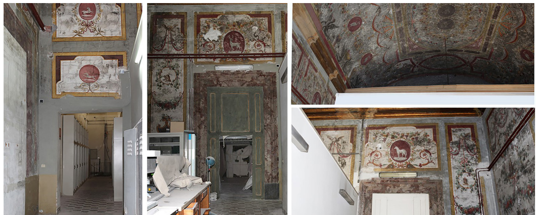
Fig. 4. Interior views of the Theater, which is now occupied by superfetation used for archives, with an evident state of decay for the wall decorations.
