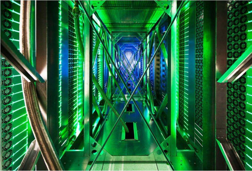
Fig. 2: White Space, Google Data Center Server Room, Mayes County, Oklahoma, USA. Source: https://www.google.com/intl/de/about/datacenters/gallery/#mayes-county-server-aisle , protected by copyright
