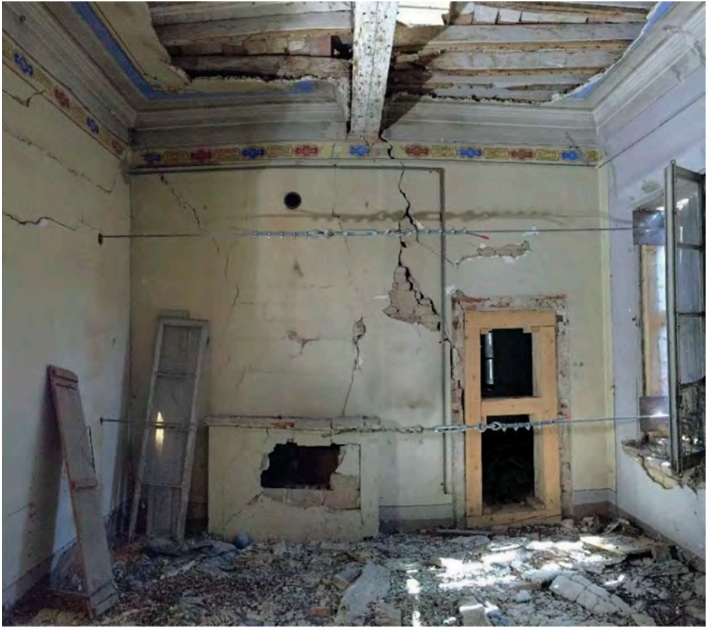
Figure 9. The critical condition in west wing's first floor with deep masonry cracks, partial collapses of suspended ceilings. In the foreground are the chainings for safety measures.
