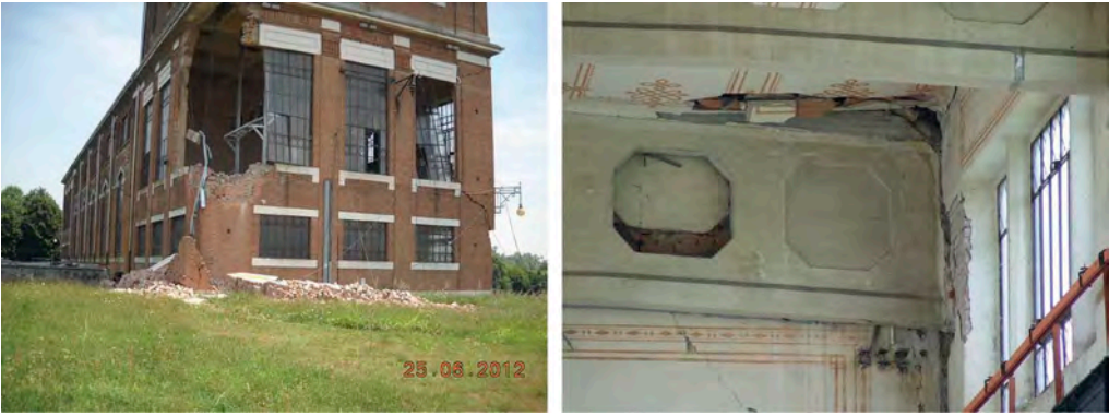
Figure 7. Mondine dewatering station, collapse of an angle of the turret and, at right, damages of the Vierendel beams supporting the floor of pumps room.
