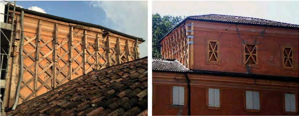
Figure 6. Safety operations by the Fire Department to preserve the central tower and the building from possible structural collapse.
