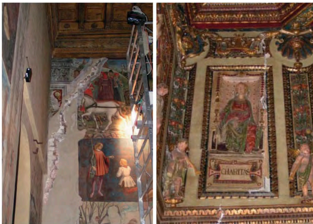
Figure 6. On the left, damages to the hall of the months side and re-opening of the damage caused by the 1570 earthquake. On the right, detail of the damage to the Vice and Virtute side.
