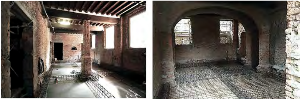
Figure 24. The construction of ventilated structural crawl spaces at the foundations. In correspondence with the wall-cutting sheath present along the entire perimeter, wall continuity was restored with the application of bidirectional glass fibre mesh.
