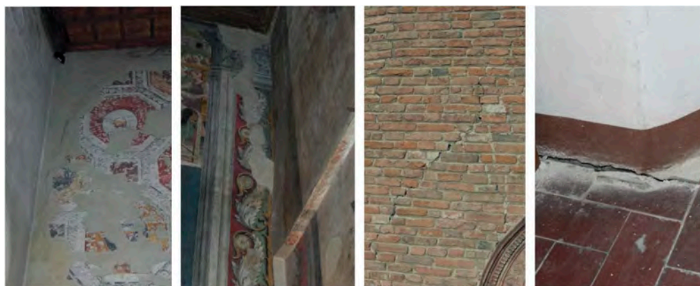
Figure 12. The reopening of old cracks and the formation of new ones.
