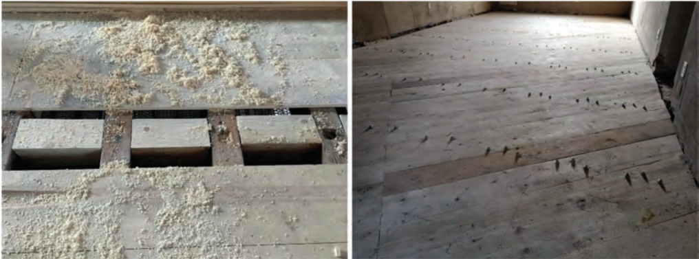
Figure 16. Insertion of wooden beam segments in the extrados between the rafters - Stiffening and consolidation of slabs by means of triple planking and connectors.
