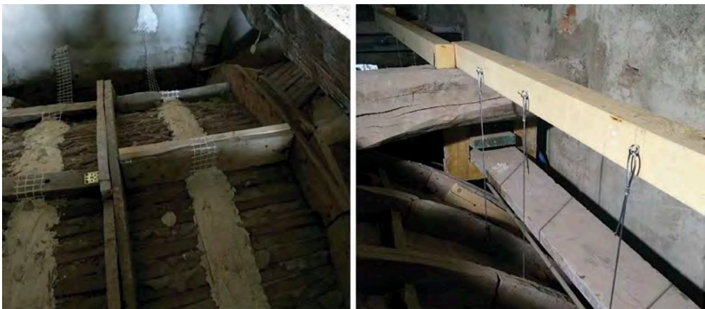
Figure 26. Images of the restoration of the wooden structures of the decorated vaults. In addition to some meticulous replacements of completely rotten elements, some doubling of the structures was carried out with new anchors, safety restraints with steel hangers and fibre matting with lime-based adhesion promoters.
