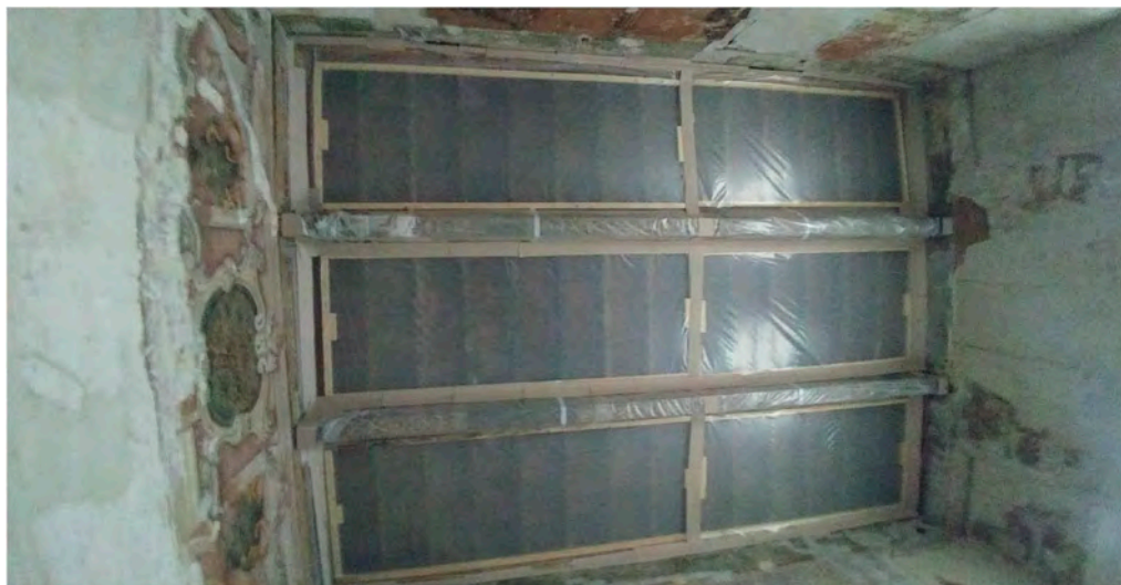
Figure 11. Hall on the main floor with structures in wood and panels in non-woven fabric and plastic material, created to protect the decorated wooden slab.
