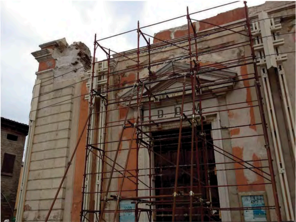
Figure 4. The first phase of securing the Church of San Felice: the scaffolding framework to prevent the overturning of the walls.
