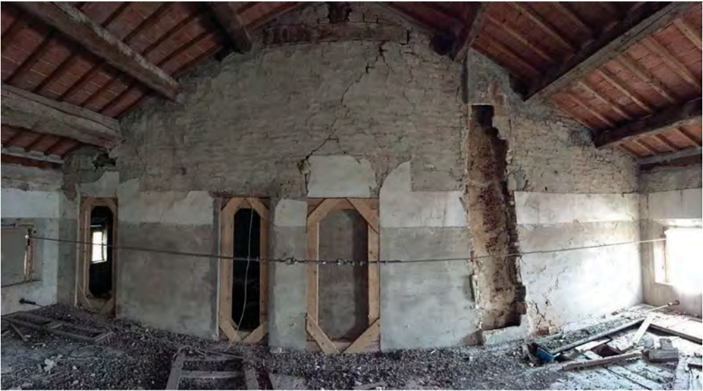
Figure 16. The condition of the rooms in the attic of the western body, which had been uninhabited for decades, was such that even accessing them during the survey was very difficult.
