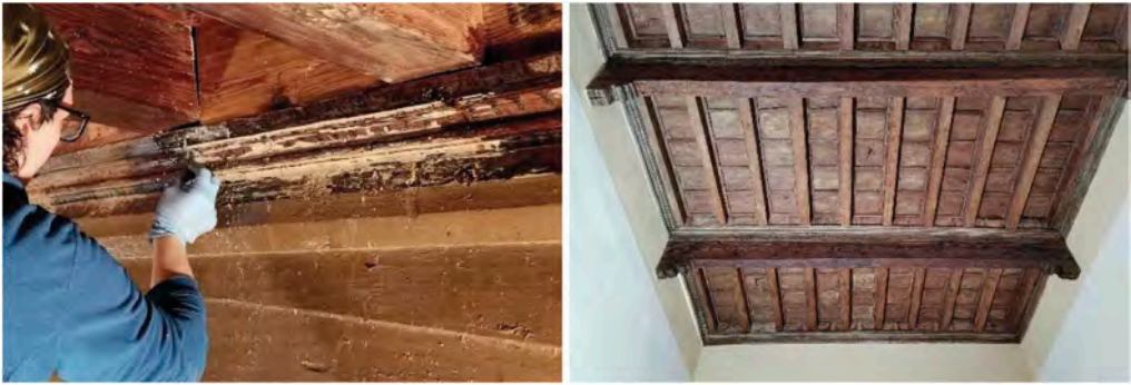
Figure 27. Restoration of the wooden slabs on the ground floor of the 15 th -century part.
