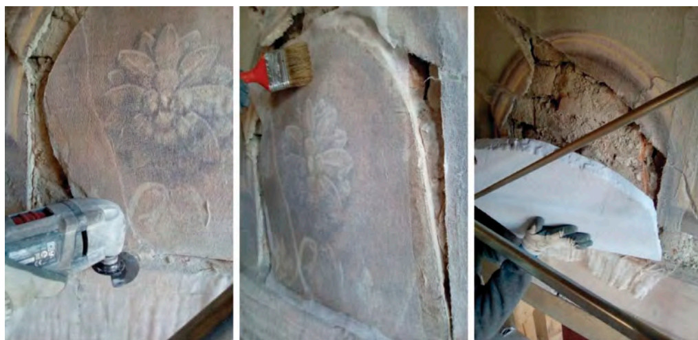
Figure 22. The pictures show the sequence of securing the decorations by sticking gauze and tissue to prevent any detachment of the decorated plaster. Micro-cutters, whose low vibration and absence of rotating blades ensure maximum precision, were used to cut the plaster. Laying the panels and cataloguing. In the panels, the 'back' of the decorated detached piece can be seen.
