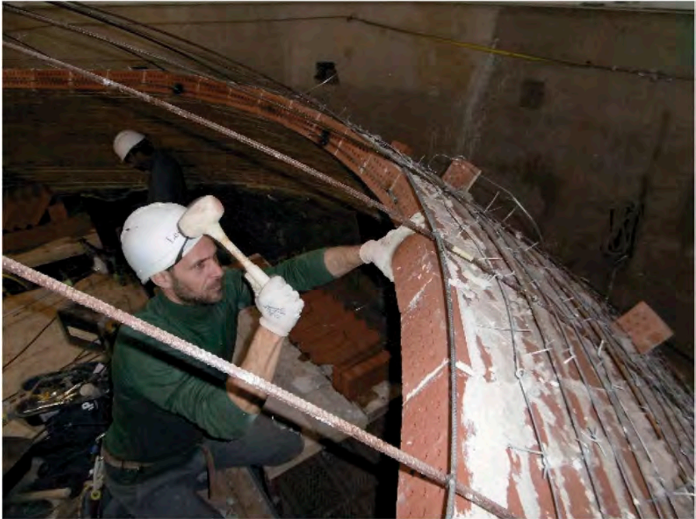
Figures 14-15. The phases and methodology of the construction: extradossal rib made of metal rods and laying of the brick elements from inside the wall cap under construction.
