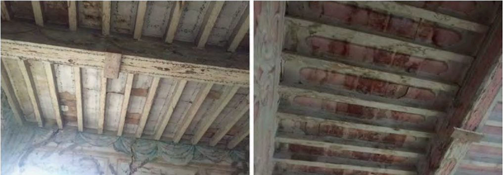
Figure 15. The rooms on the first floor of the western enfilade have wooden ceilings with lime-washed brick tiles and fine decorations that echo the motifs on the walls. There is evidence of water leaking from the roof as a result of the earthquake.
