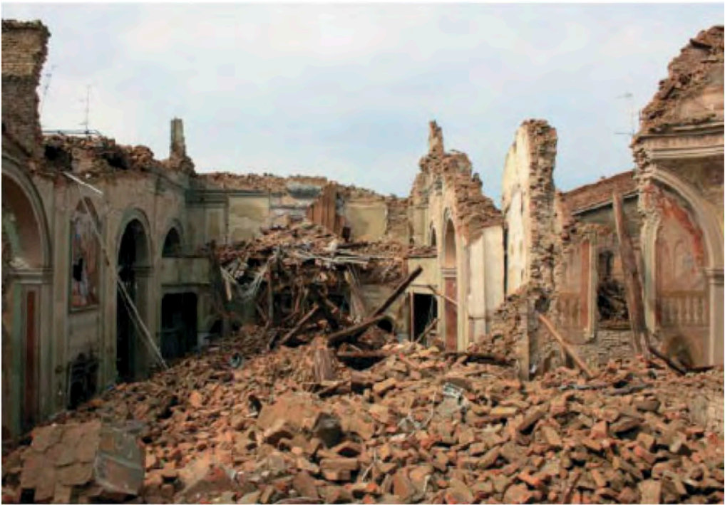
Figure 3. The parish church of San Felice sul Panaro following the 2012 earthquake.
