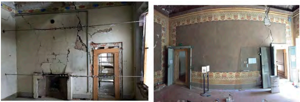
Figure 10. Some pictures of the rooms on the first floor of the west wing. The earthquake damage also caused large infiltrations of rainwater.
