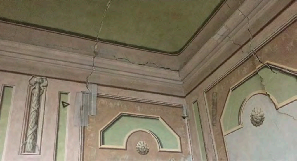
Figure 12. The decorations in the rooms on the main floor of the main body of the building were seriously damaged.
