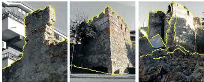
Figure 15. Walls of Durrës, serious damage into crenellations.
