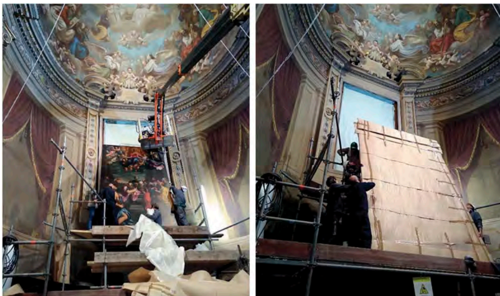
Figures 19-20. Securing operations by the fire brigade with the supervision of a MiC official personnel.
