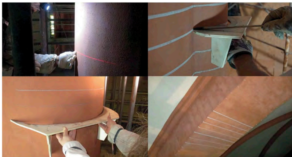
Figure 15. After tracing with a laser level and using shapes and templates with variable curvature to follow the splay of the columns, a pictorial reconstruction of the decorative draft on columns and arches was established using lime paints.
