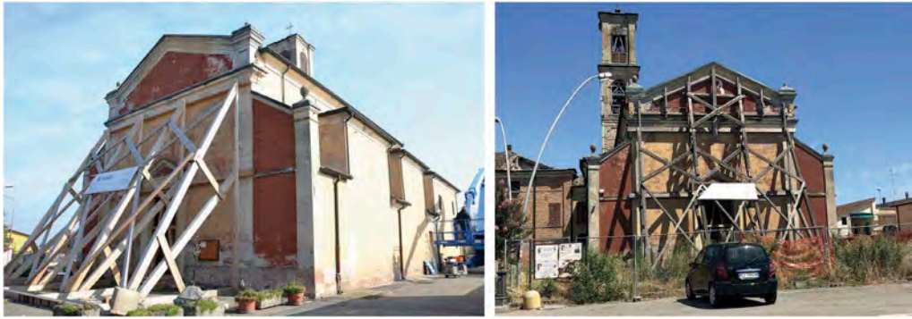
Figure 3. San Michele Arcangelo Church in Bomporto (MO): on the left the wooden rakers installed in 2012, on the right the worsened conditions of the same interventions in 2019.
