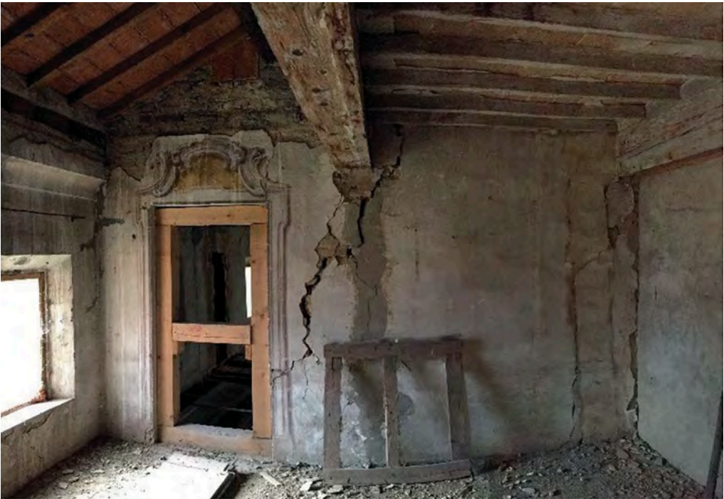
Figure 17. Partial collapses of floors and unsafe portions of the roof represented the main difficulty.
