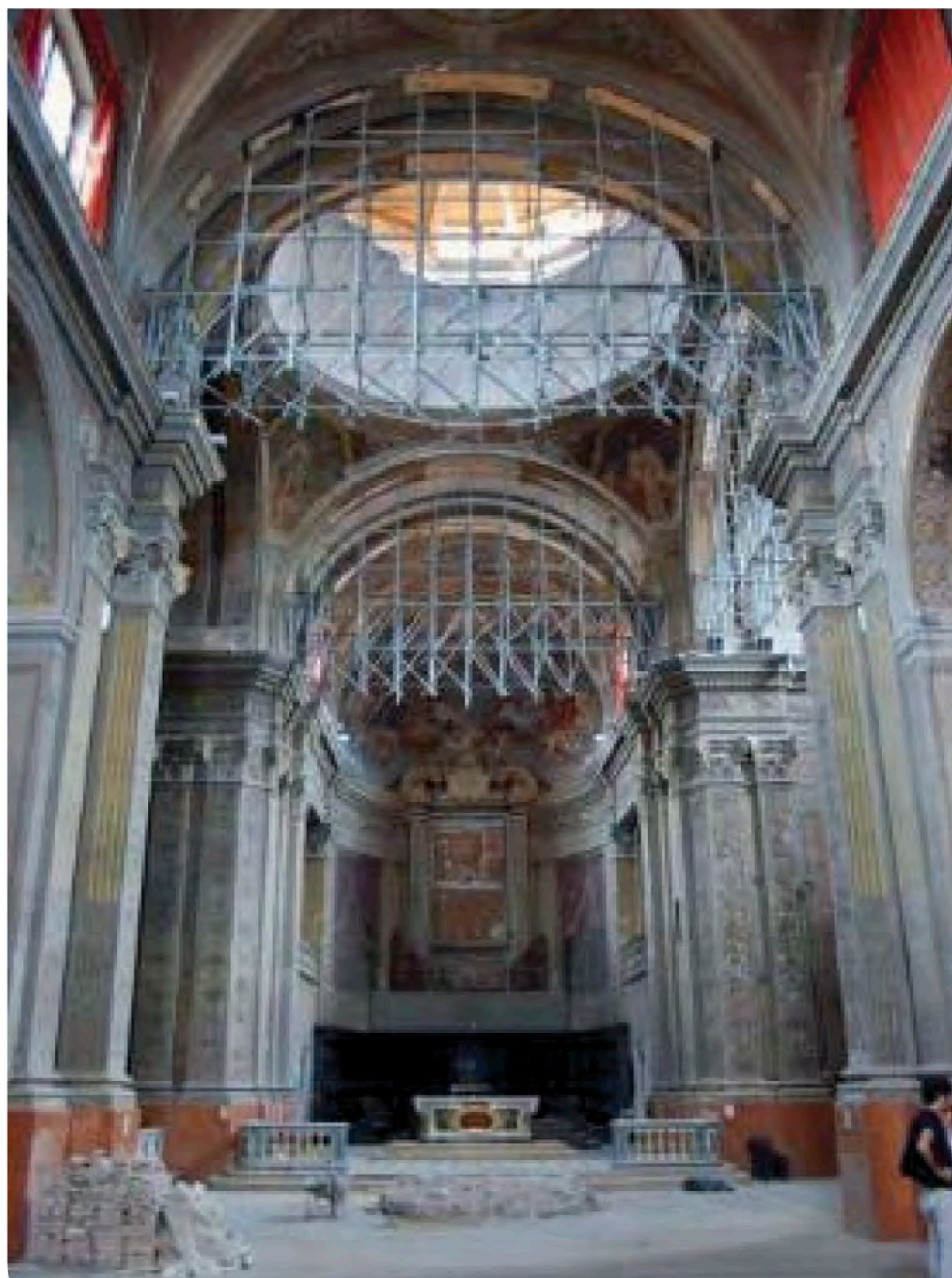
Figure 10. Picture of the interior of the church after the removal of rubble and the construction of temporary structures to support the walls in the area around the central dome.
