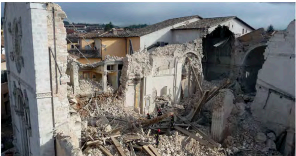
Figure 10. The Basilica of San Benedetto in Norcia following the 2016 earthquake.
