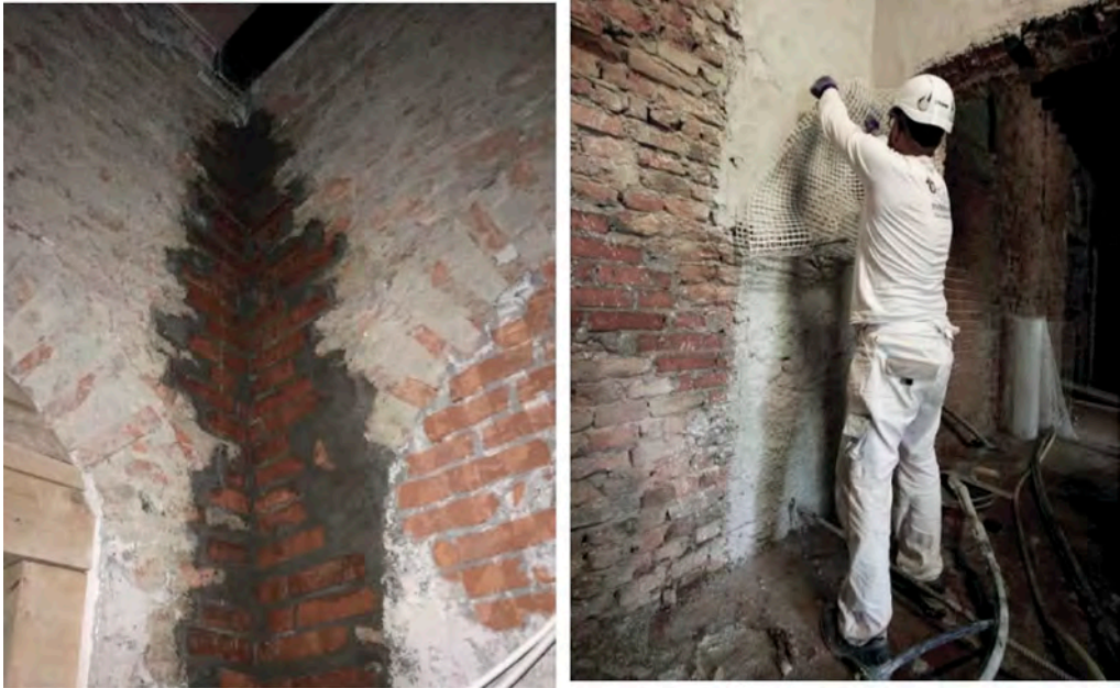
Figure 23. Several masonry walls had little or no toothing between corner walls. Two types of intervention are envisaged, angular like-for-like replacement or the laying of fibreglass fabrics, also placed at an angle, on lime-based adhesion promoters.
