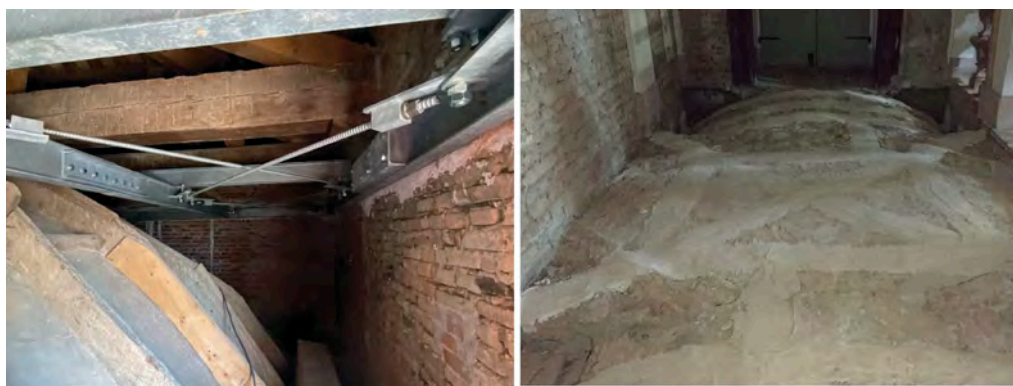
Figure 27. Images of structural reinforcements on the intrados of the vaults. A large two-dimensional steel girder lattice will make any movement of the central tower's masonry more difficult.
