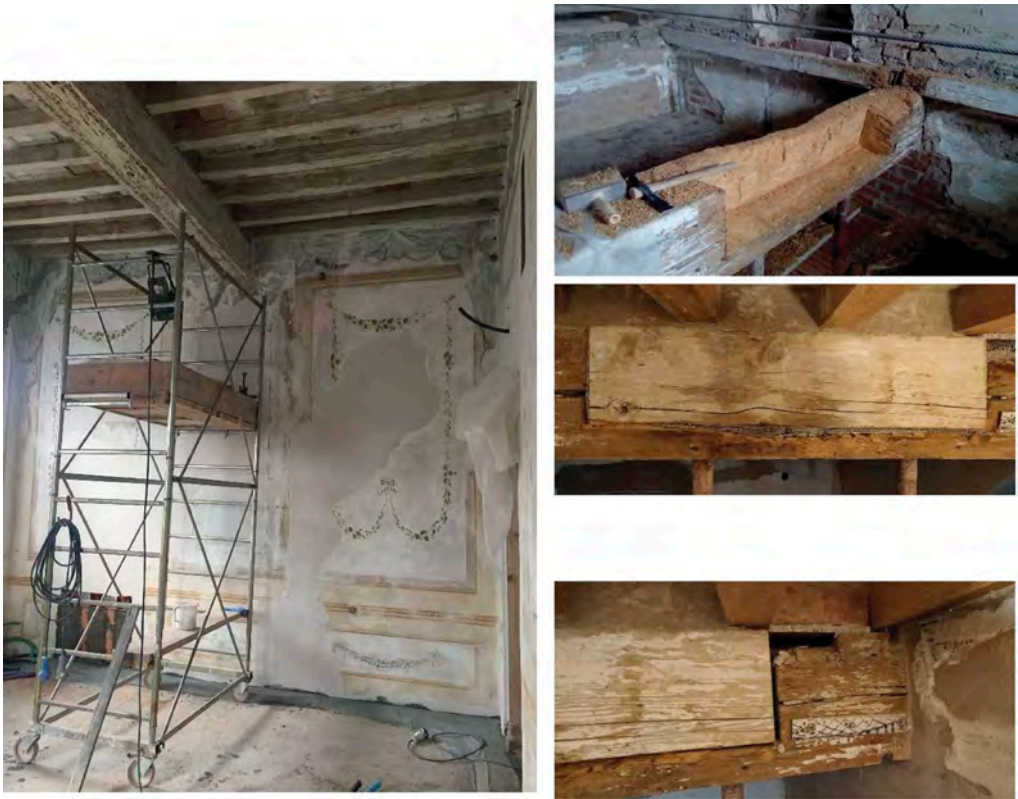
Figure 25. Prolonged exposure to the weather and parasite attack completely damaged a painted wooden beam head in one of the rooms on the main floor of the west wing, requiring the insertion of a wooden prosthesis. The rotting area was removed by carefully cutting down to the healthy part of the beam. The prosthesis of the same wood species was prepared and fixed with wood screws and threaded stainless steel bars.
