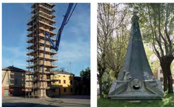
Figure 6. On the left, Sant'Anna in Reno Centese (FE): the isolated bell tower was heavily damaged by horizontal cracks and requires emergency action for restore adequate safety conditions to get close to the building. On the right, Santi Senesio e Teopompo Church in Medolla (MO): in order to prevent the overturning of the bell chamber, the macro-element was removed and conserved in a storage area.
