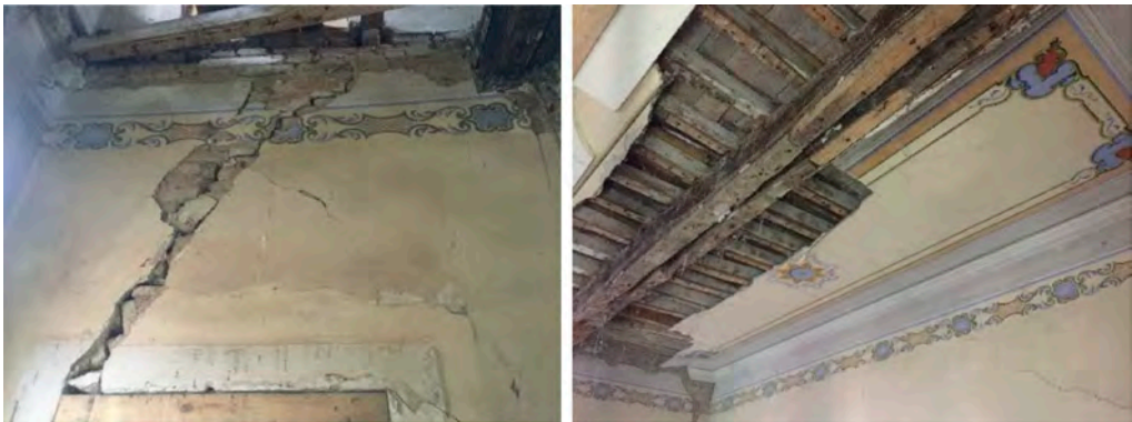
Figure 8. The first floor of the west wing was in a very critical condition, with deep cracks in the masonry, partial collapses of the suspended ceilings and widespread rotting of the wooden beams.
