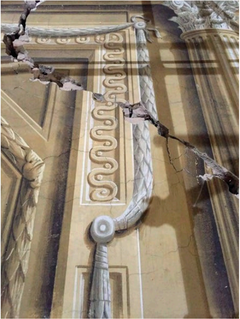
Figure 13. In one of the cornices of the Sala Centrale, the earthquake damage caused the decoration to shift by almost 10 cm.
