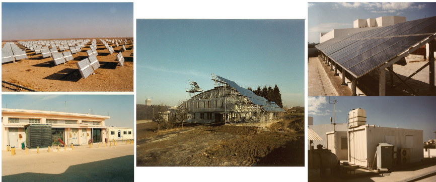
FIGURE 2.1 The three solar-hydrogen production facilities manufactured and operated as part of the German–Saudi Arabian HYSOLAR program, 1986–1995. Left: 350/500 kW solar-hydrogen production demonstration plant in Riyadh, Saudi Arabia (operated 1993–2000). Center: 10-kW-solar-hydrogen R&D facility in Stuttgart, Germany (operated 1987–2004). Right: 3-kW-solar-hydrogen test facility in Jeddah, Saudi Arabia (operated 1989–1995).
