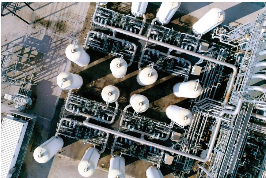
FIGURE 17.5 Top view of Air Products' CO 2 VSA trains used to remove more than 90% of the CO 2 contained in the reformer PSA feed gas. Credit: Air products.
