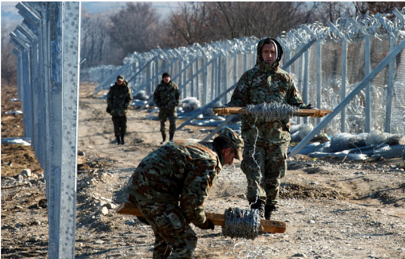
Figure 7-11 Barb-wired wall on the Greece-North Macedonian border.
