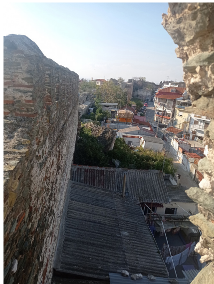
Figure 17. Wall houses in the upper town of Thessaloniki often used as temporary shelter by people on the move.
