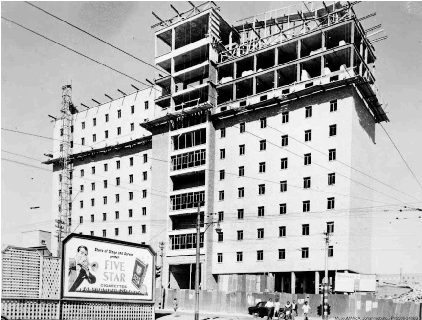
FIGURE C.2 John Vorster Square under construction, Johannesburg, 1968. Photographer unknown Image courtesy of South African History Archive/Museum Africa
