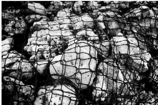
Figure 3.11 Closeup of the Furanfushi breakwater. Expensive plastic-coated galvanized steel mesh was used for the installation less than a year before, and already the steel is starting to rust. Such structures rarely last more than a year or two before collapsing and needing to be rebuilt. (Photograph by Wolf Hilbertz, 1997.)
