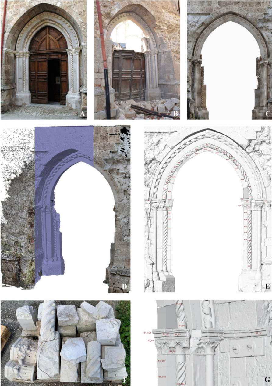
Fig. 2. Some significant images regarding the damages and the project to rebuild the side portal of the Church of Santa Maria Argentea in Norcia. In image A, a photo of the portal before the earthquake. In pictures B and C the portal after the earthquake in a view and in the orthomosaic realised through photogrammetric modelling. In image D the photogrammetric model. Image F shows the portal fragments in storage. Images E and G show the reassembly of the catalogued pieces.
