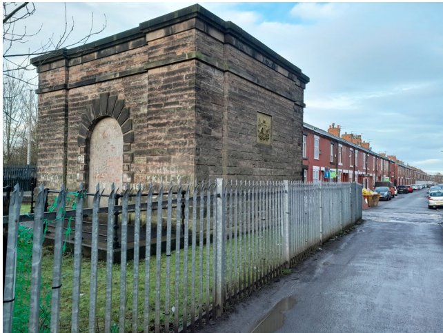
Fig. 5.27 Electricity substations, Brailsford Road, Fallowfield (with a plaque displaying the city's coat of arms) (Author, 2023).
