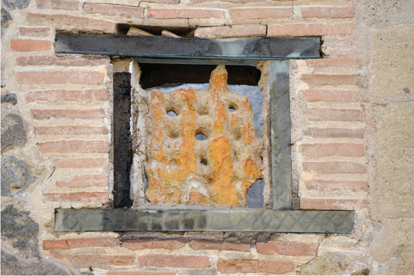
Fig. 3. Remains of a wooden window frame and iron bars (Photograph by Carole Raddato, July 2014, via Wikimedia Commons, cc by-sa 2.0.)
