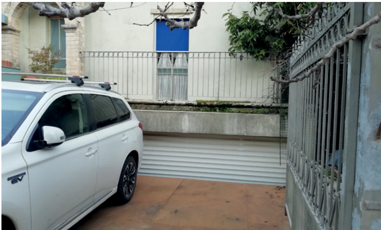
Figure 8.13 Fake, inaccessible garage door. The underground space designated for a garage has been illegally merged with the main house. Location undisclosed. © Rachele Alterman.
