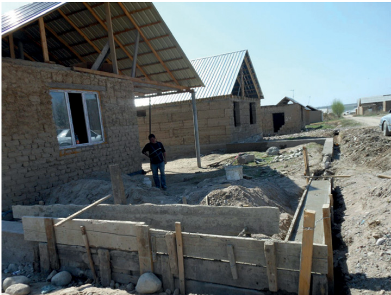
Figure 5.2 Laying the foundation of a future house in Ak Zhar. © Eliza Isabaeva.
