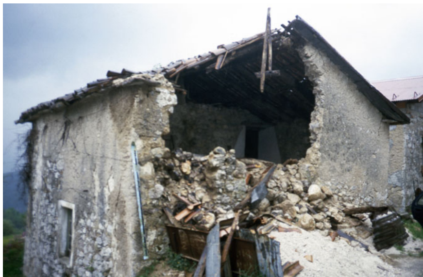
Fig. 10.7 Damage to buildings in Drežniške Ravne after the 1998 earthquake. Photograph Matija Zorn
