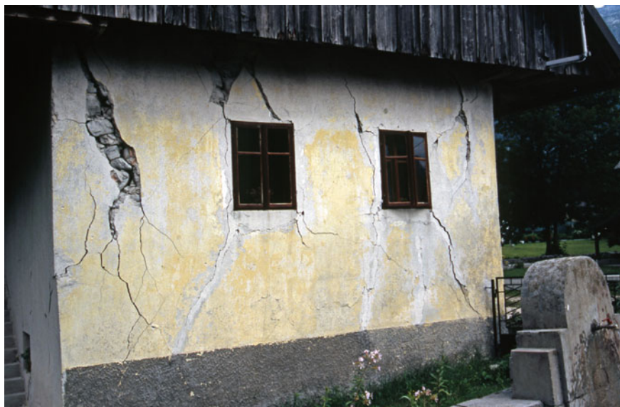
Fig. 10.8 Damage to buildings in Čezsoča after the 2004 earthquake. Photograph Matija Zorn
