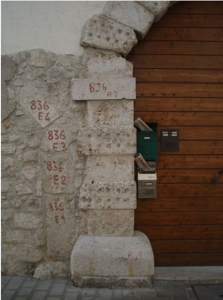
Fig. 10.3 Markings based on which buildings were reconstructed after the 1976 earthquakes are still visible on many buildings in the old town of Venzone. Photograph Primož Pipan
