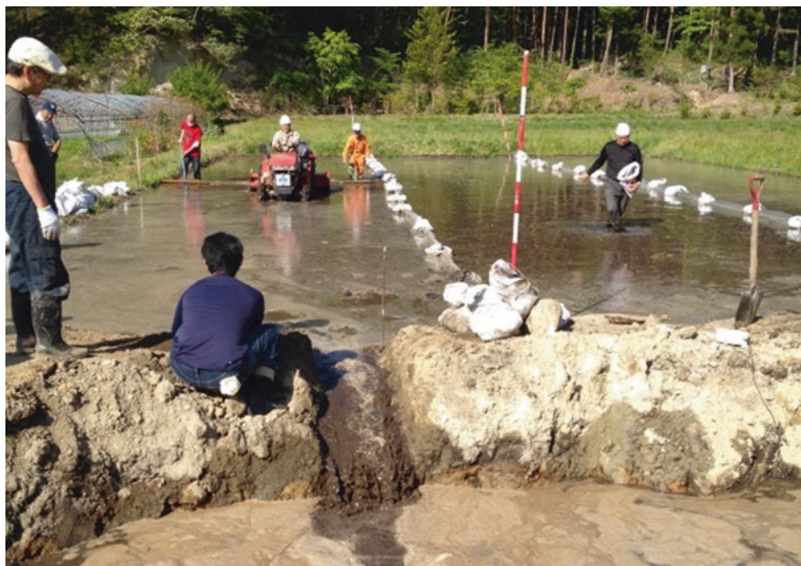
Photo 16.2 Decontamination of farmland by muddy water flushing out method with a tractor
