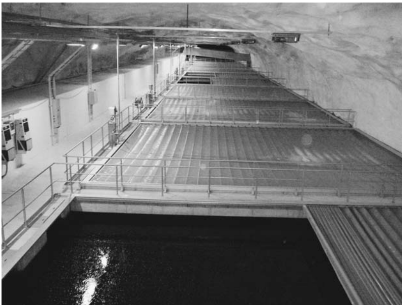
Figure 16.4 Viikinmäki Waste Water Treatment Plant is built underground. The figure shows biological post-filtration. Source: Photograph Rajala, 2007.
