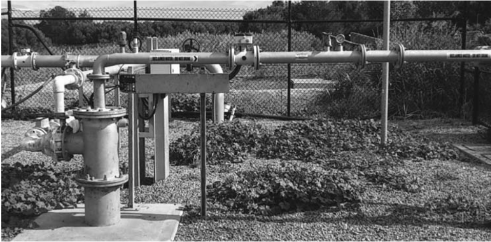
Figure 6.1 Managed Aquifer Recharge injection pump at Greenfields Wetlands, Salisbury. Source: Photograph May 2012, Carol Fort.
