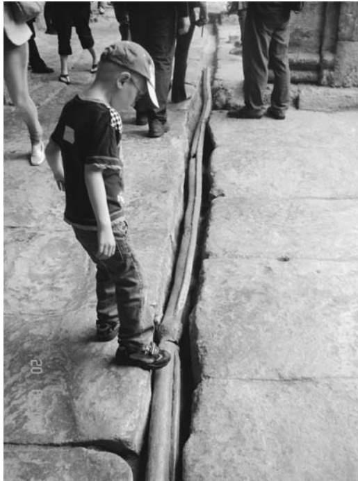
Figure 8.1 Lead pipes were commonly used water distribution lines in antiquity, as in the Roman Aquae Sulis, situated in modern Bath, Britain.
