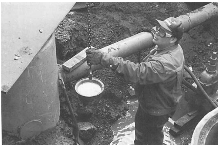
Figure 8.2 Making a connection in an old steel pipe using molten lead in Tampere in 1998. Source: Photograph P. Juuti.
