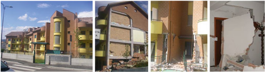
Fig. 14.22 Left : the dwelling building complex (3 buildings) of Via Borgo dei Tigli 6-8-10 in L'Aquila (Pianola area), which had been just completed before the 2009 Abruzzo earthquake. Right : damage caused to the building by this event
