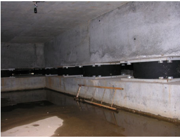
Fig. 14.13 Some of the 193 HDRBs, manufactured in Italy, which protect the building of Fig. 14.12 (picture taken on September 23, 2011, during the 2011 Sochi Conference) (Martelli et al. 2012a)
