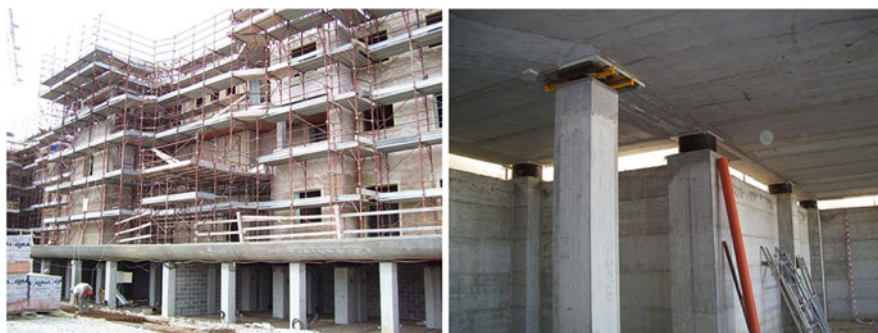
Fig. 14.24 Left : seismically isolated dwelling building complex under construction in Ozzano Emilia (Bologna), irregular in shape (61 m \times 28 m; 2 buildings with 2 staircases, connected to the second floor; 4 isolated above ground isolated floors, with the isolators installed in the non-isolated basement). Right : some of the isolators of the building (61 HDRBs and 56 SDs)
