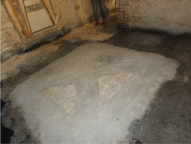
Fig. 15.7 Reinforcement of a cross vault with strips of FRP laid at the extrados
