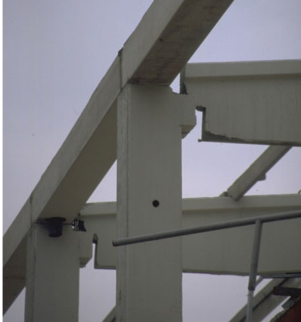
Fig. 4.13 Displacements are typically very large
