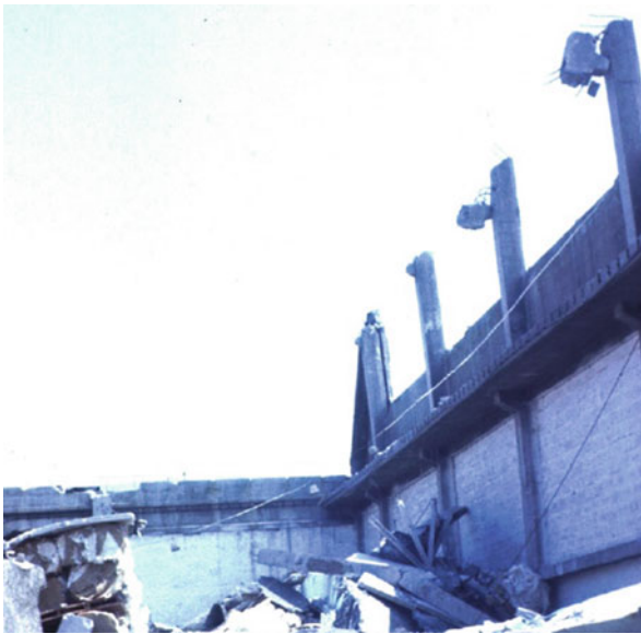
Fig. 4.12 Collapse of the roof system during Montenegro earthquake due to soil effects and poor connections
