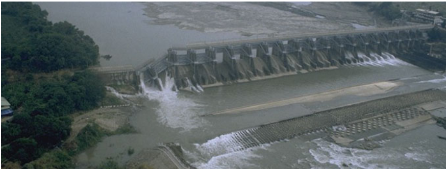
Fig. 20.2 Failure of two openings of the Shih-Kang weir caused by fault movements during the 1999 Chi-Chi earthquake in Taiwan
