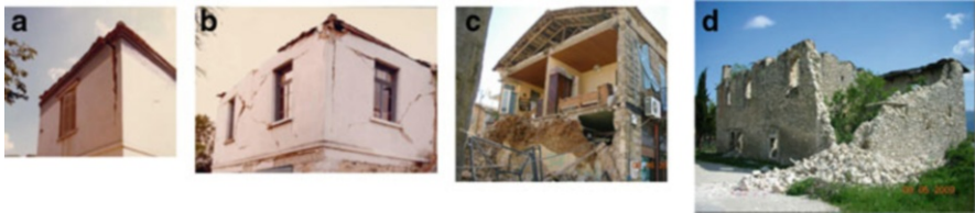
Fig. 8.13 Typical damages due to out-of-plane seismic actions. (a) Typical vertical crack due to out-of-plane bending of the solid wall. (b) Typical vertical crack at mid-length of the wall and separation of walls at the corner of the building. (c) Out-of-plane collapse of wall. (d) Collapse of the corner of a building (due to combined in-and out-of-plane action)
