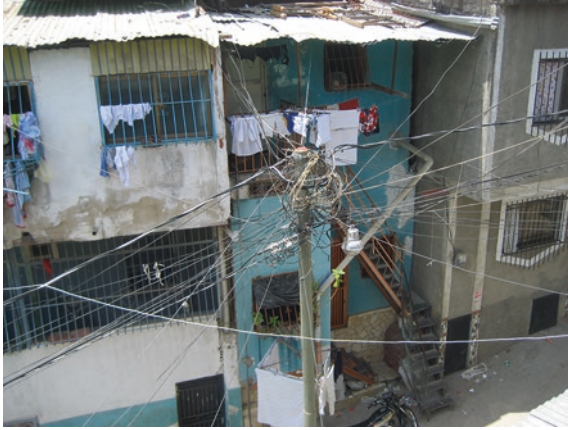
Photo 1 Typical electricity pole in informal neighborhoods. Photo by the author
