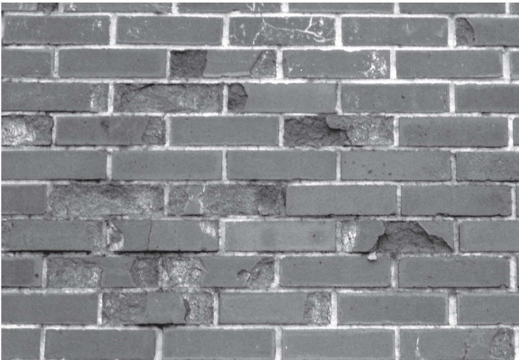
Figure 10.3. Surface Deterioration from Sub-freezing Consistently Moist Brick.
