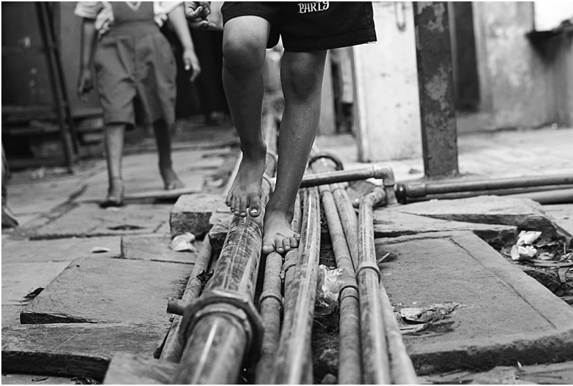
FIGURE 9. Shared water lines, Mumbai. Water lines run just above the surface of Jogeshwari's alleys.
