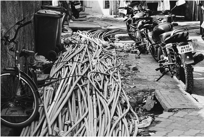
FIGURE 16. Water lines serving Premnagar. Some of these lines are legal; others are illegal. It is difficult for engineers (or anyone else) to tell them apart.
