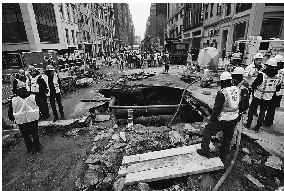
FIGURE 17. Workers at the site of a break in a 137-year-old water main in the Greenwich Village neighborhood of New York, January 16, 2014. Photo by Ozier Muhamad/ New York Times /REDUX.
