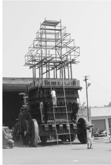
Figure 5: Construction of the upper part of the chariot, Belur, KA. Photo: Cristina Bignami
