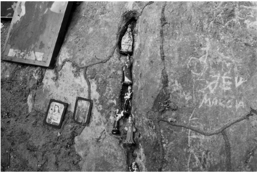
■ Figure 22 Cracks in the Wall, Milagre de São Roque, Bahia, 2007
