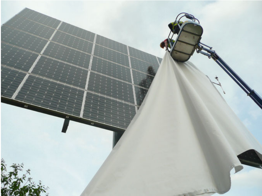
Fig. 15.12 SunBeam . Installing the temporary screen on the solar tracker, UCLan, Preston, May, 2011. Copyright © Chris Meigh-Andrews, 2019
