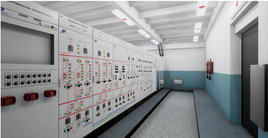
Fig. 19.8 3-D model of the main control room
