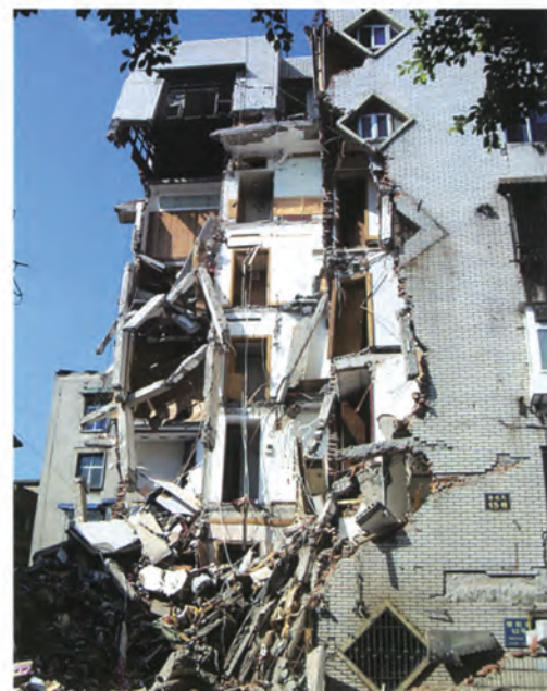
▲ Collapsed building in the town of Guangji
