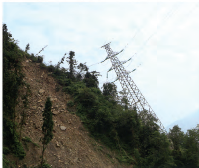
Collapsing high-voltage wire transmission towers
