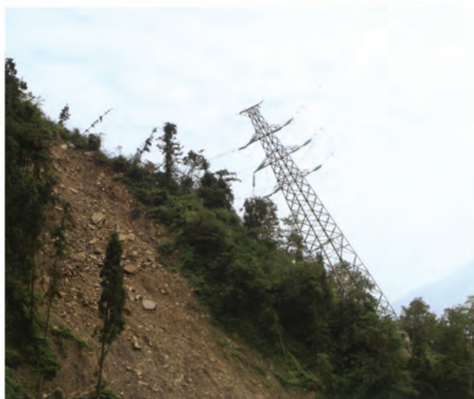
Collapsing high-voltage wire transmission towers
