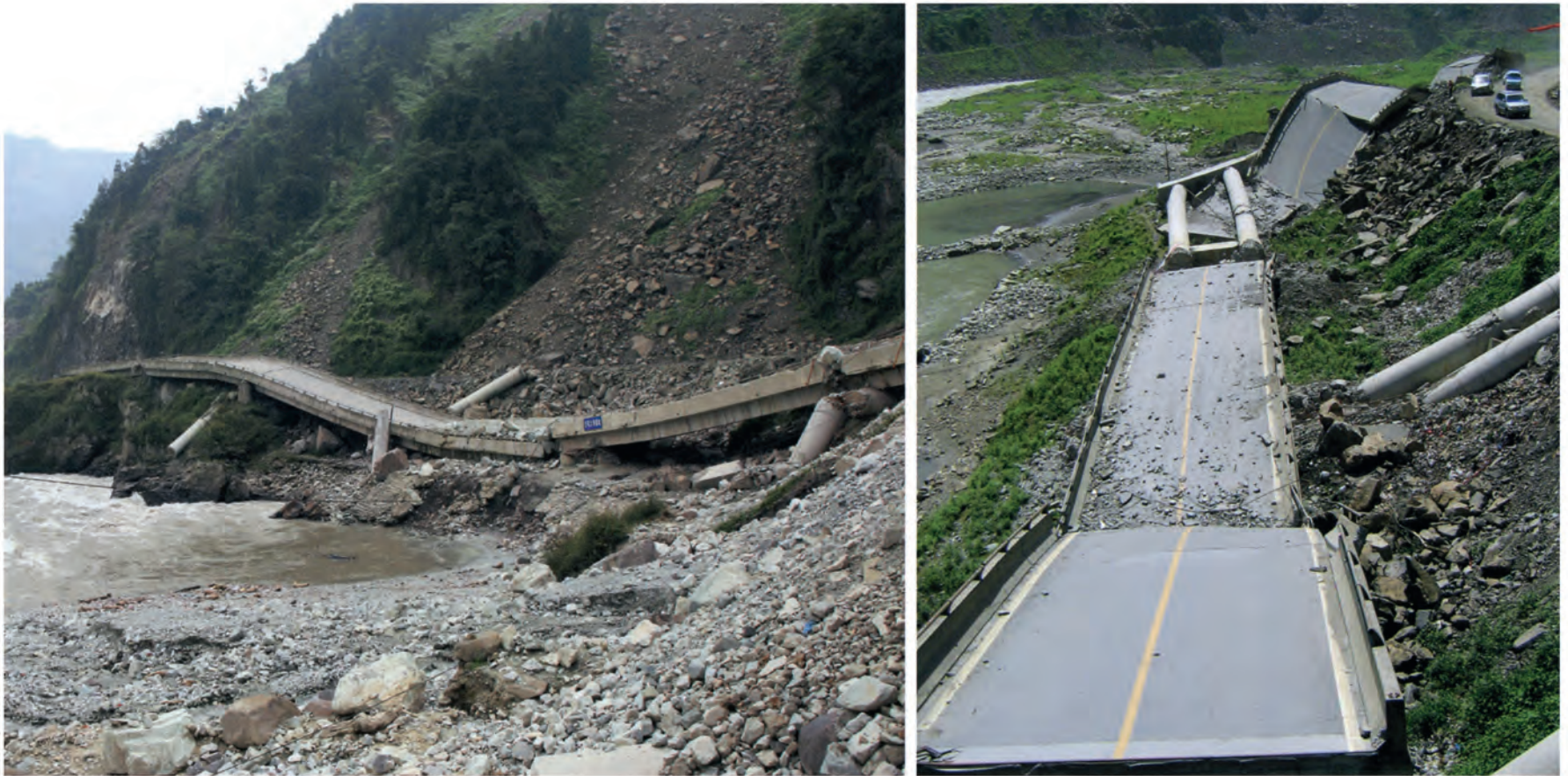
Post-earthquake photos of Baihua Bridge
