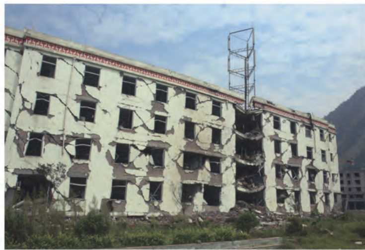
A building destroyed by the earthquake
