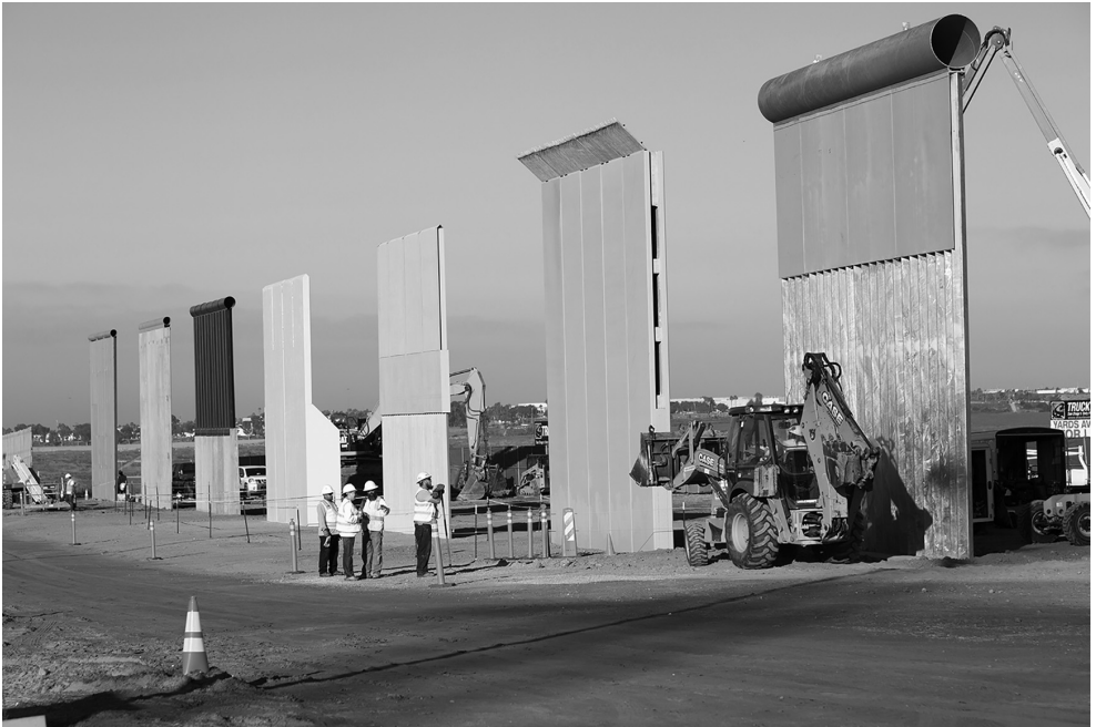
Figure 9.10 Ground views of different border wall prototypes as they take shape during the Wall Prototype Construction Project near San Diego.
