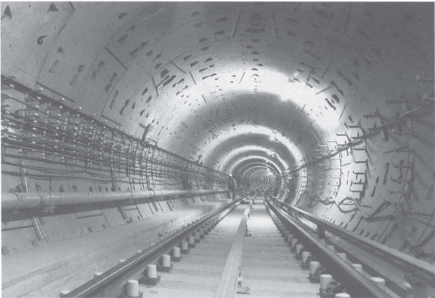
8. Typical completed tunnel for the Jubilee Line extension (photo courtesy of QA Photos/Jubilee Line Extension Project).
