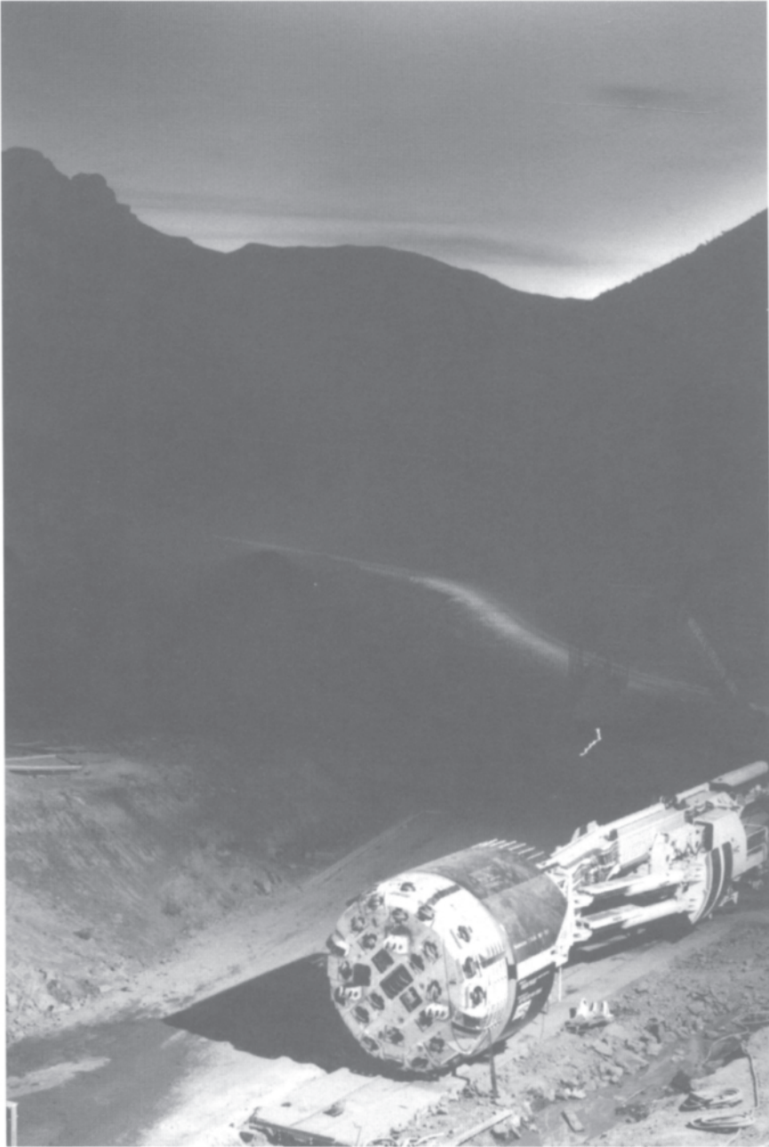
4. Robbins 5 metre diameter TBM with back-up ready to start 17.5km drive for the 45km long Lesotho Highlands transfer tunnel (photo courtesy of QA Photos Ltd).
