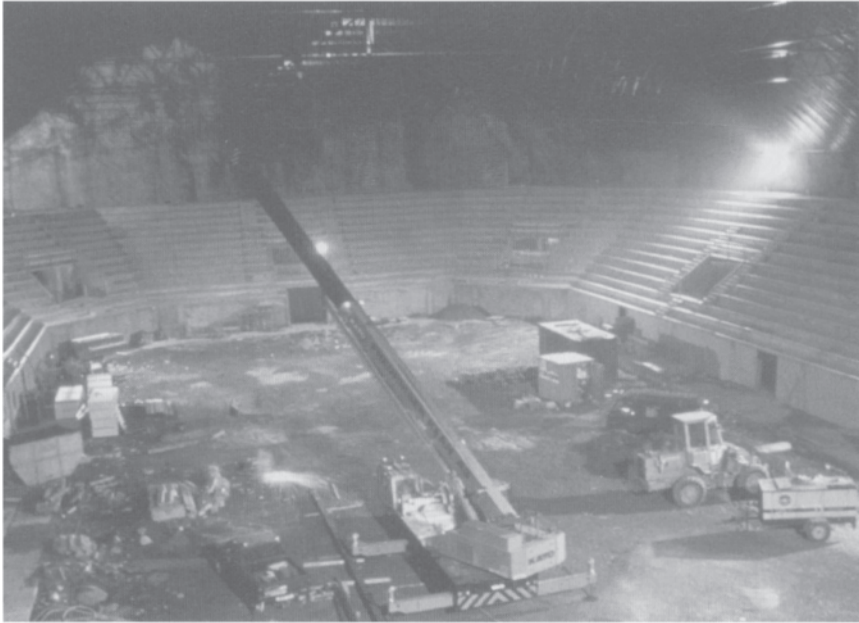
1. Gjøviksports cavern for 1994 Winter Olympics in course of construction. The main cavern has a span of 61 metres, height of 25 metres (photo © Scan-Foto Hans Brox).
