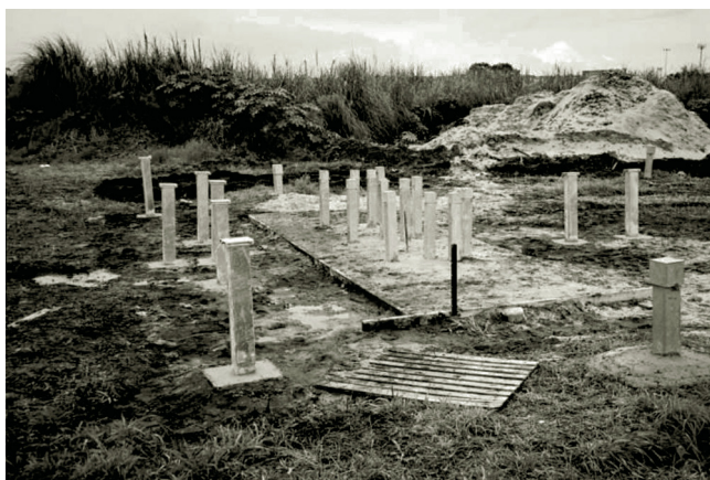
FIGURE 12.9 The completed pilot-scale reactive iron barrier with a protective concrete cap. (From Orica Ltd.)
