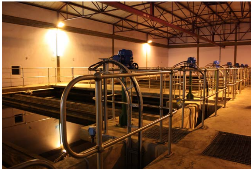
Views of process units of the New Goreangab Plant in Windhoek.
