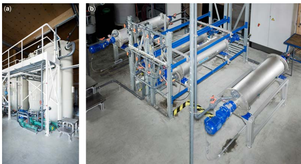
Figure 7.4 View of the wastewater treatment: left photographs, from left to right: equalization tank, sedimentation tank, bioreactor (water) and rotating disk filters at the right photographs.
