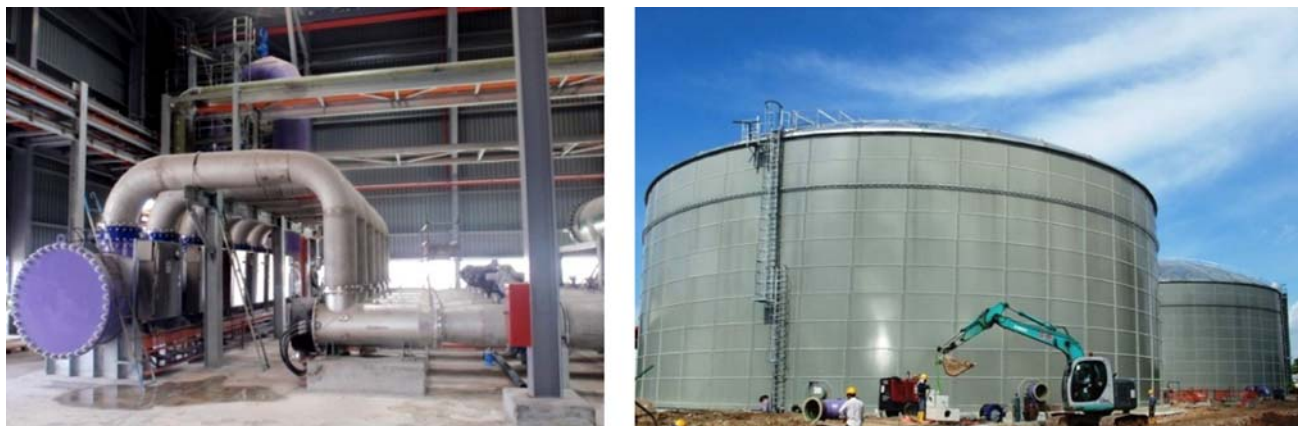
Figure 3.6 View of UV disinfection and NEWater storage tanks.
