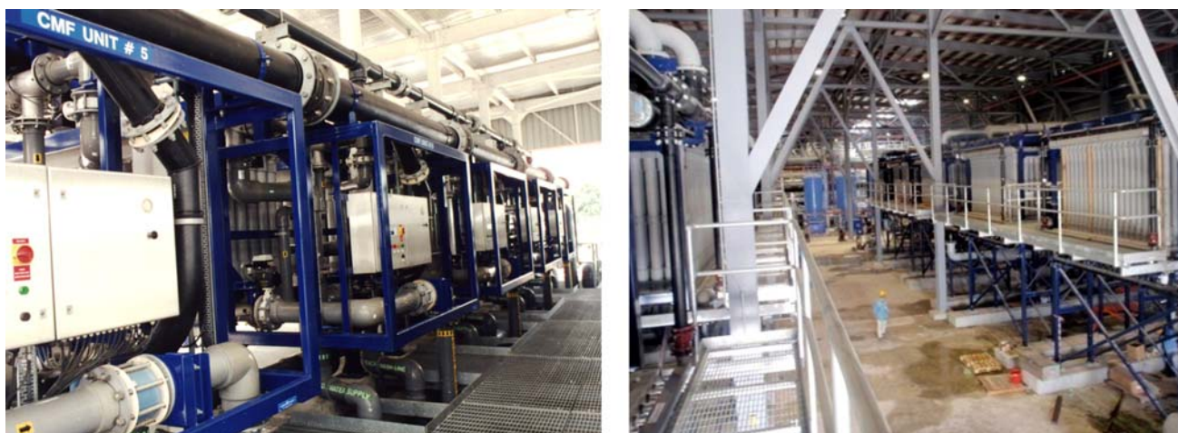
Figure 3.4 NEWater production process: view of microfiltration.
