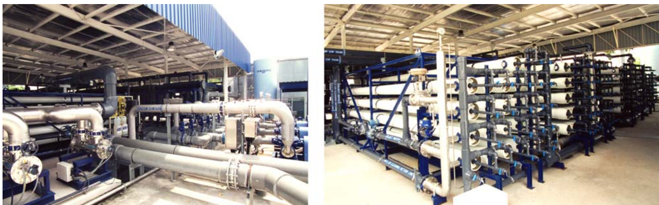
Figure 3.2 Views of the Bedok NEWater demonstration plant.
