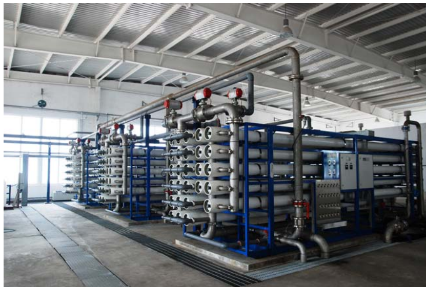
View of the reverse osmosis (RO) technology used to control recycled water salinity in Tianjin.
