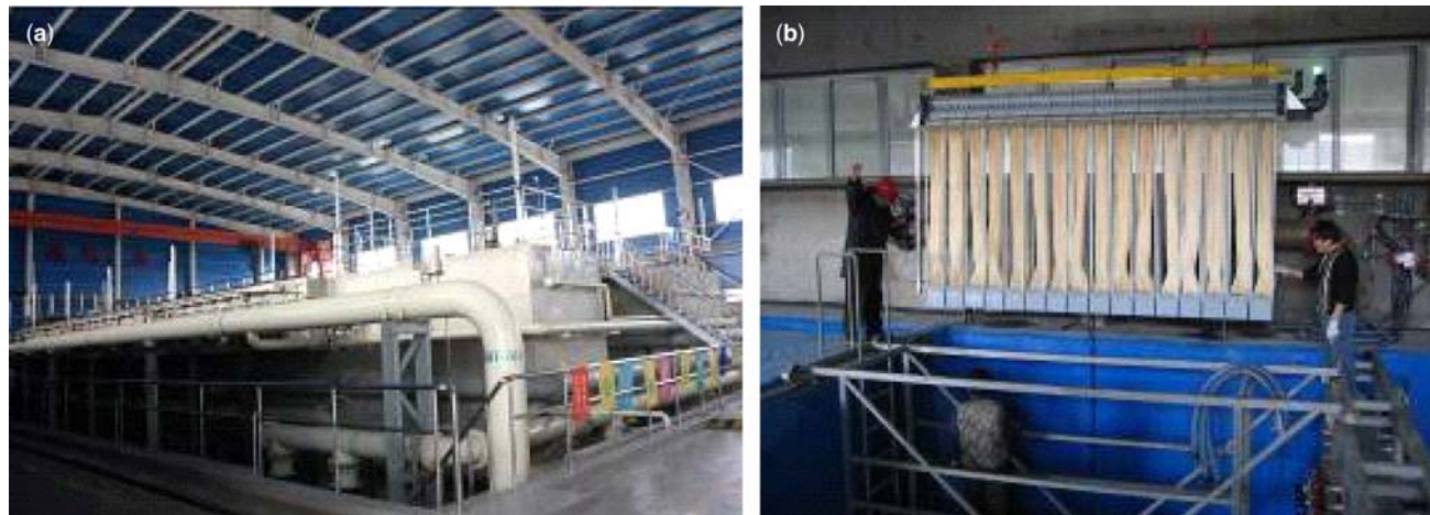
Figure 23.4 Views of the QingHe water reclamation plant (a) and the BeiXiaoHe water reclamation plant (b). (a) Tertiary filtration – ZeeWeed 1000 membrane tanks (b) MBR – installation of a Memcor Memjet module.
