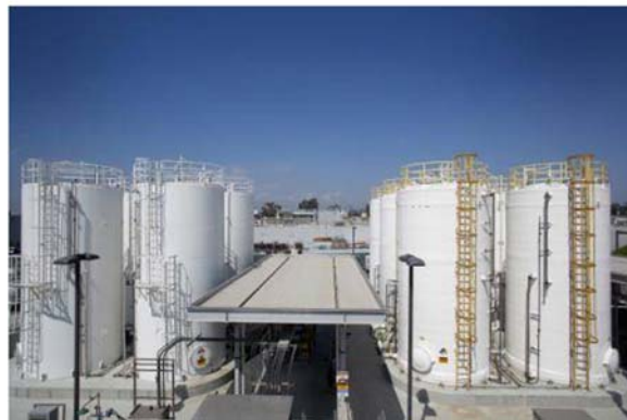
Views of the Advanced Water Purification Facility.
