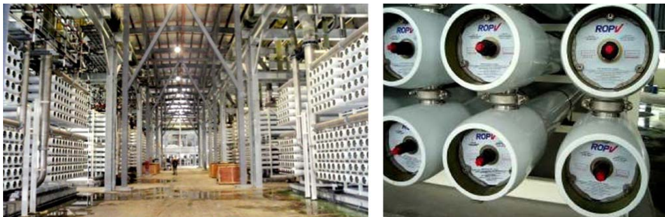
Figure 3.5 NEWater production process: view of reverse osmosis.
