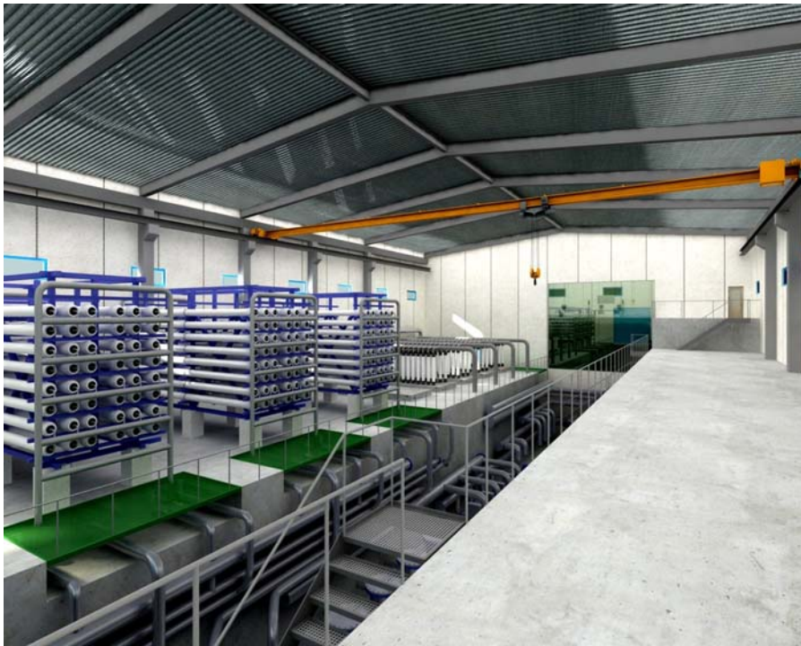
View of the advanced reclamation facility using ultrafiltration hollow fiber membranes and two-stage reverse osmosis to produce high quality recycled water for the Holmen Paper industry.
