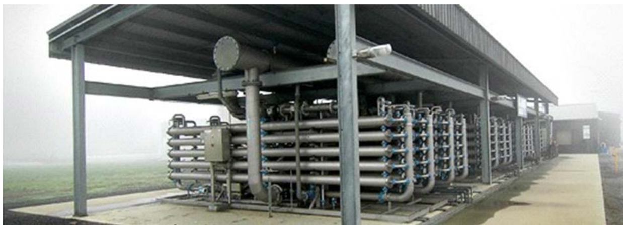
Figure 17.1 View of the ultrafiltration water recycling plant, eastern irrigation scheme (Photograph courtesy of Water Infrastructure Group, Melbourne).
