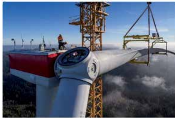
Figure 5. Installation of wind turbine blades on the tower in Gaildorf (Credit: Max Bögl (Holger Hessenthaler)).
