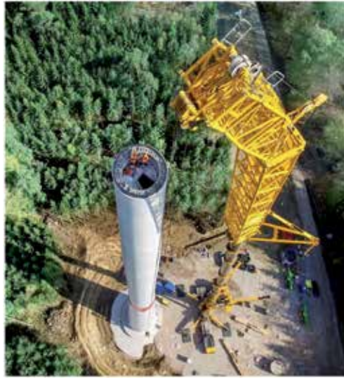
Figure 9. Installation of the internal steel tower by means of a crane (Credit: Max Bögl).
