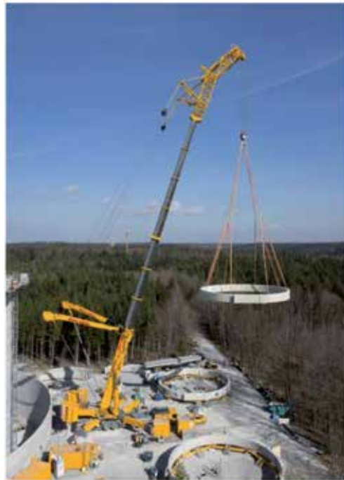
Figure 7. Putting together concrete rings at the construction site by means of the Liebherr 630 EC-H70 self-erecting slewing crane (Credit: Liebherr Plant Ehingen GmbH).
