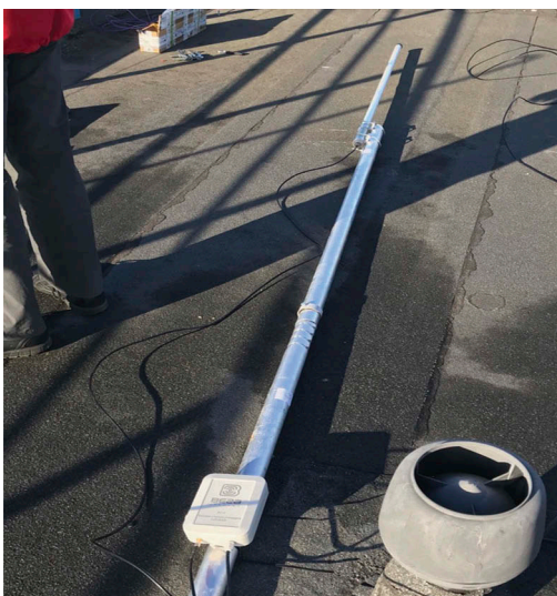
Figure 2. LoRaWAN gateway and antenna.
