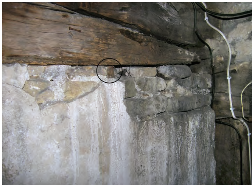
Fig. 7.25: 33 Strand Street (House 83), panel below tiebeam of north truss in hall, with brick filling and short peg or wedge (circled) to hold bricks in place (S. P.)
