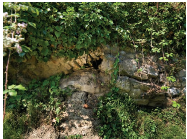
Fig. 11.14: Recently exposed brick arch on the east face of the Bulwark rampart (P. W. © English Heritage DP068602)
