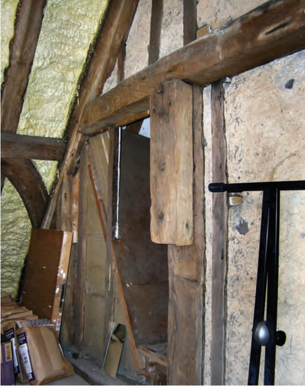
Fig. 12.47: 3 Strand Street (House 74), timber block on street face of closed roof truss at north end of the hall. It is suggested that it was put here as part of a hoist to draw goods up from the street to the left (S. P.)
