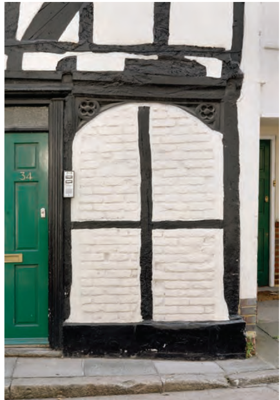
Fig. 12.17: 34 Harnet Street (30), former front doorway opening into a passage leading to the open hall behind (P. W. © English Heritage DP068595)
