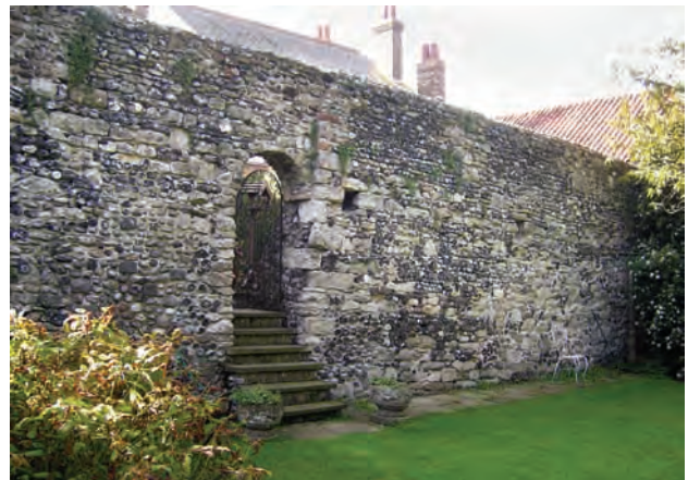
Fig. 14.3: Town wall in garden of 68 Strand Street, from north, showing possible medieval gateway (K. P. DSCN2077)
