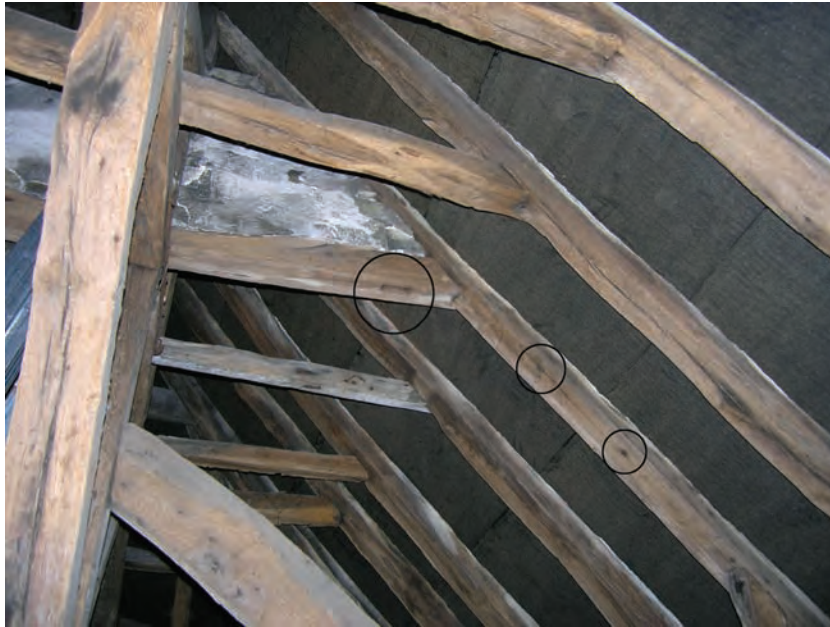
Fig. 7.24: 33 Strand Street (House 83), apex of central closed truss, east range, with brick filling still in place, and mortices (circled) for stud below collar and pegs on rafter, formerly to hold bricks (S. P.)
