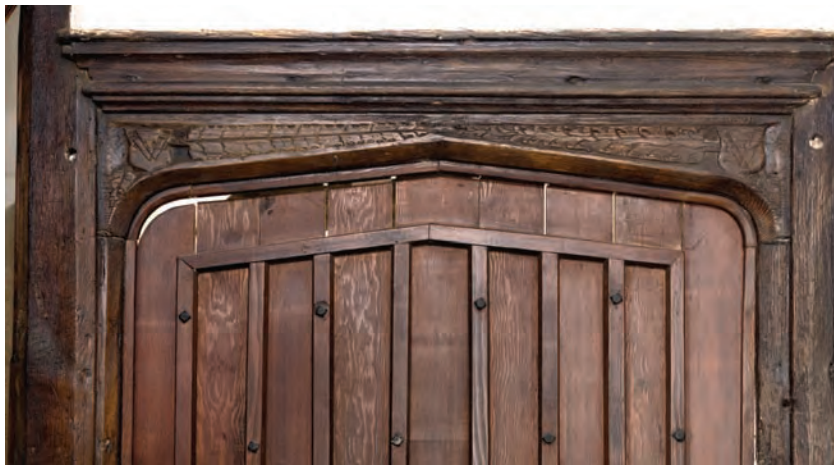
Fig. 12.32: 32 Upper Strand Street (House 98), details of doorway in cross wing (P. W. © English Heritage DP044046)
