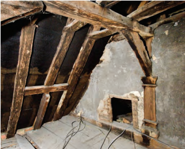
Fig. 12.16: 8 Cattle Market (House 7), top of former roof light at attic-floor level (P. W. © English Heritage DP026097)
