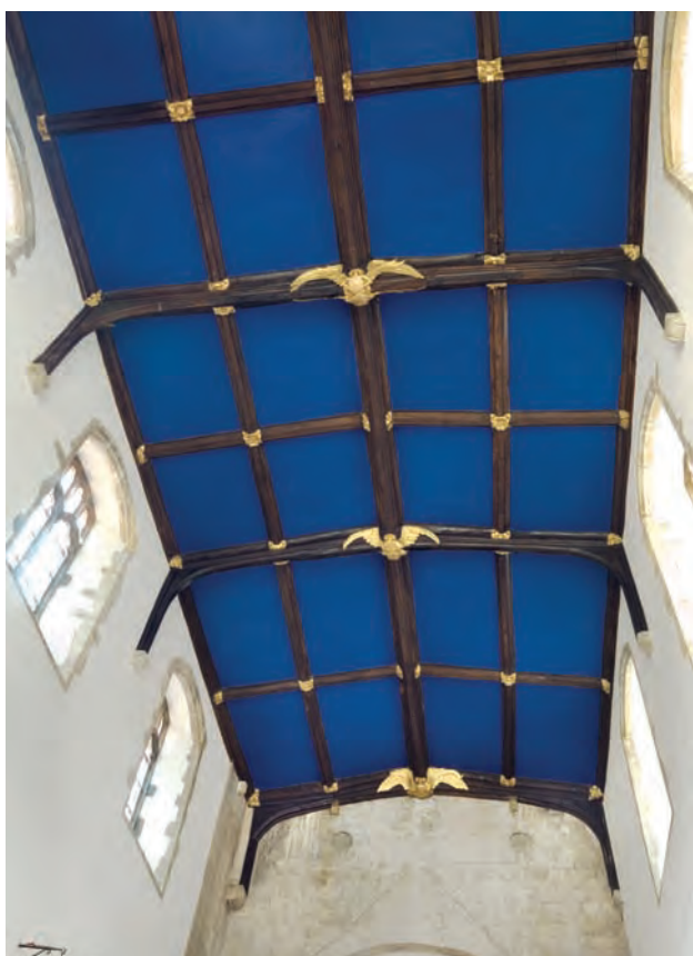
Fig. 13.2: St Clement's church, nave roof looking east (P. W. © English Heritage DP044038)
