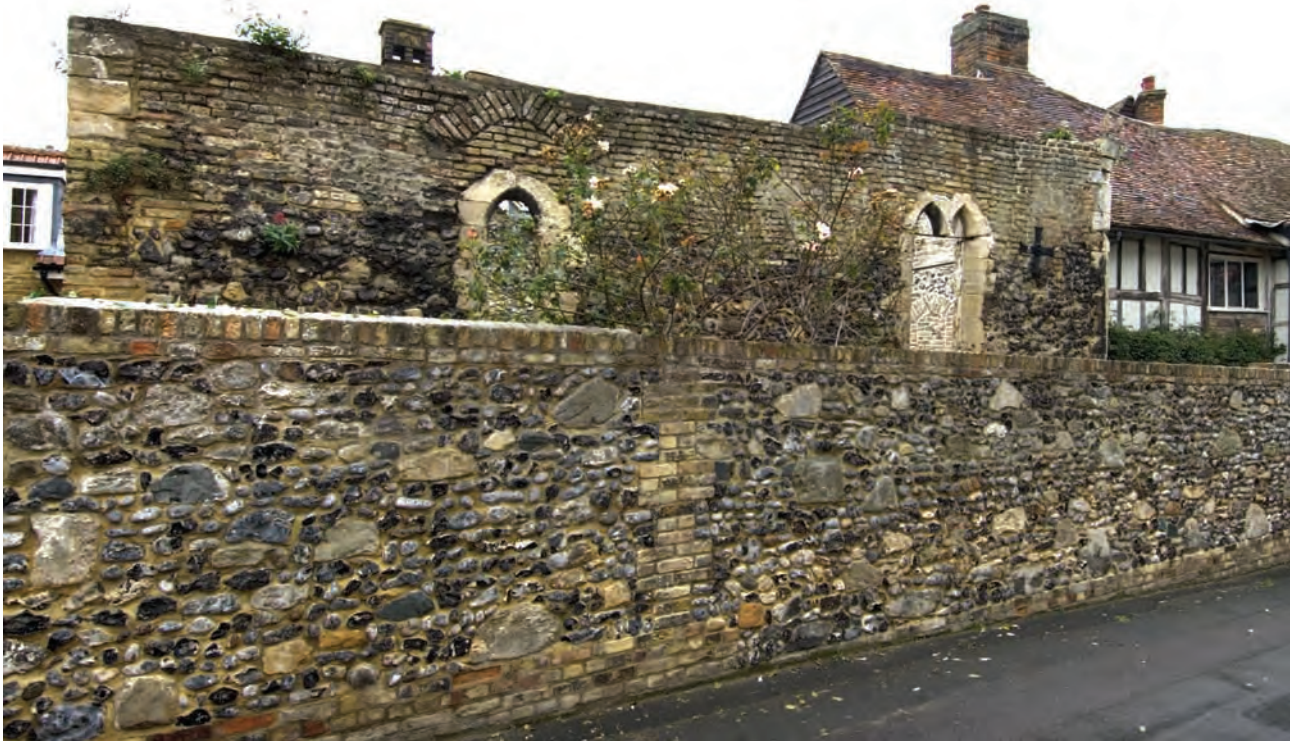
Fig. 7.13: Building in Three Kings Yard (House 78), east face of first floor (P. W. © English Heritage DP044598).
