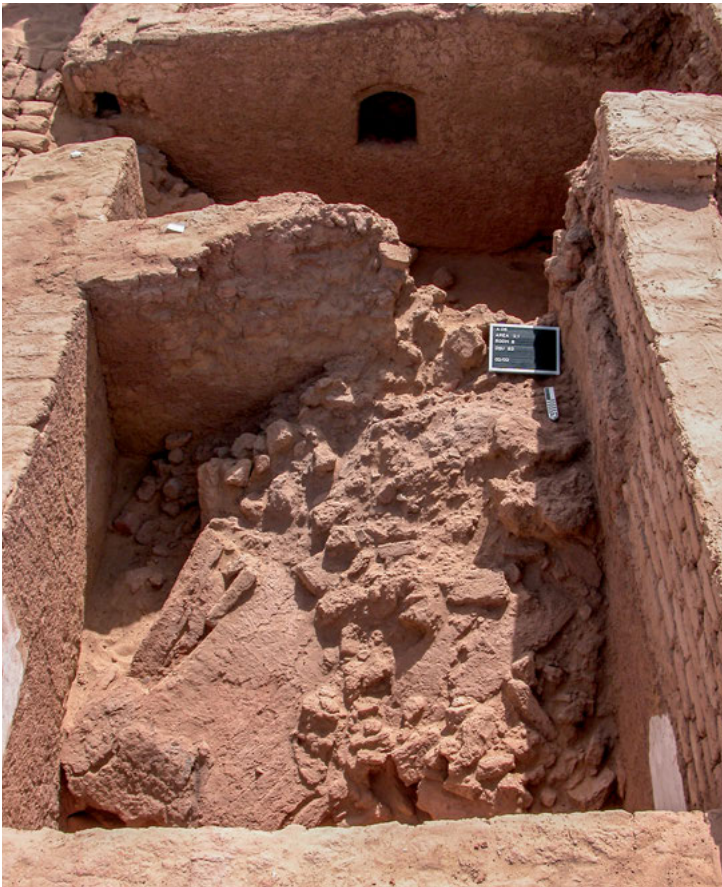
Fig. 4: Amheida: filling of room 8 in Serenos's house. The collapse of the ceiling.
