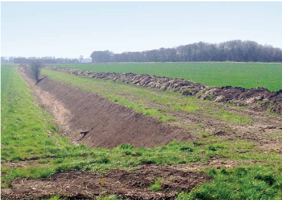
Figure 3.10. Recently dredged ditch near Skidbrooke, with spoil heaped several metres into the field. Photo: Author.
